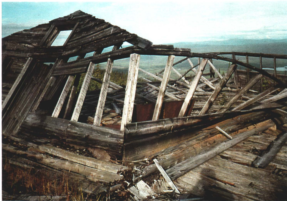
Photo 2. Delapidated wood frame structure at mine site.
