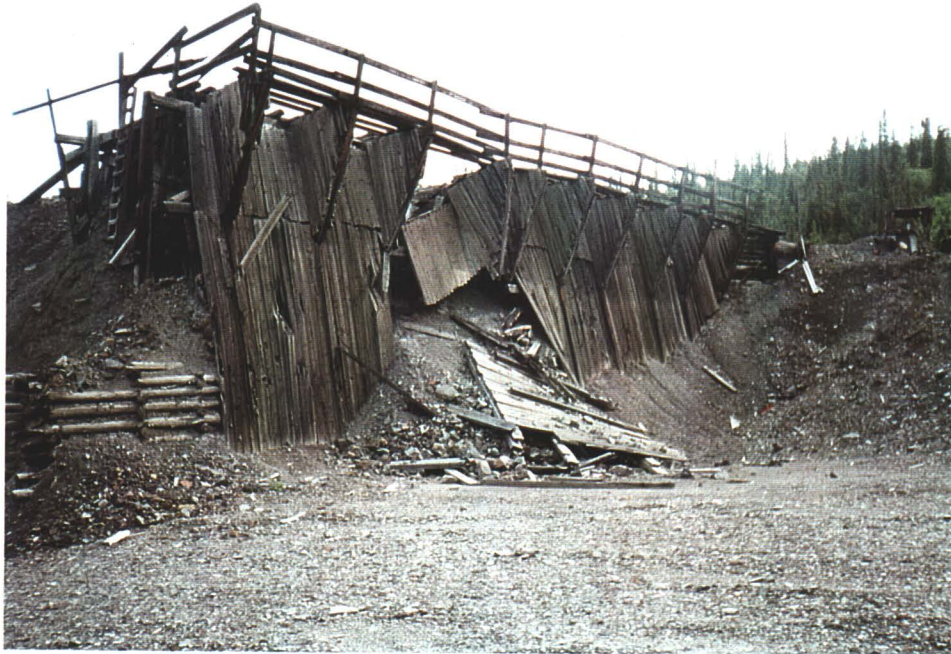
Photo 3. Deteriorated condition of load out facility necessitates expedient demolition.
