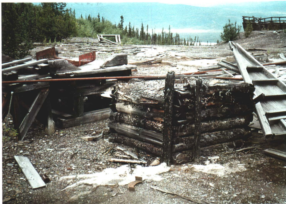
Photo 15. Damaged cribbing used to support power poles.
