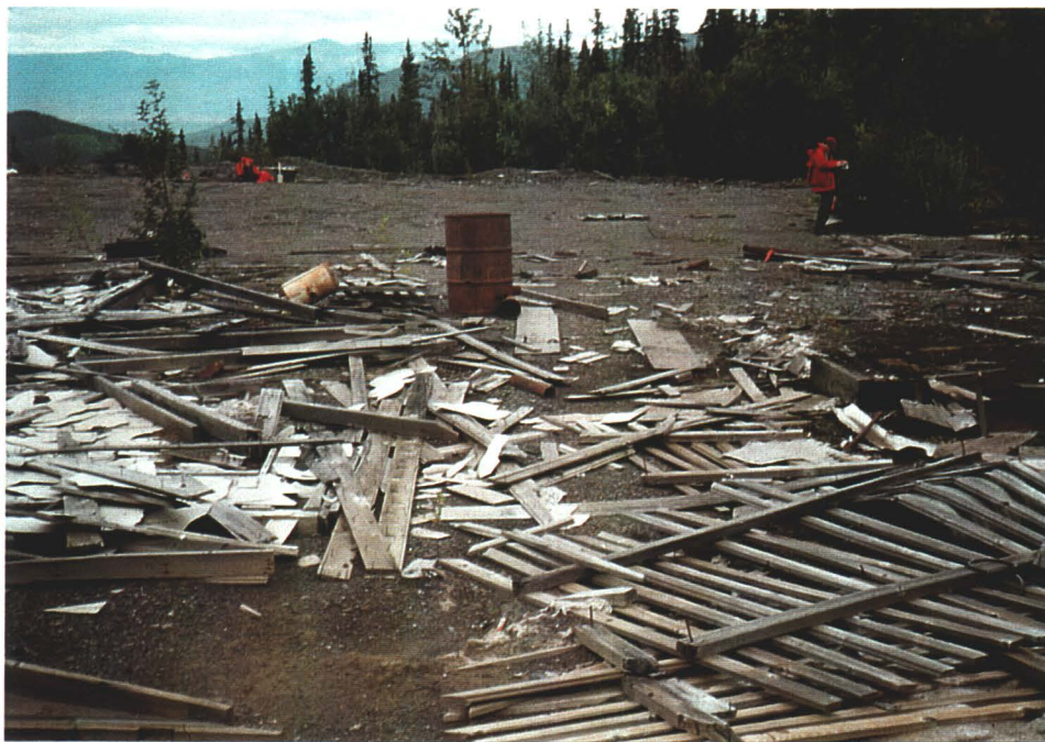
Photo 6. Residue of waste material from building collapse common to site.
