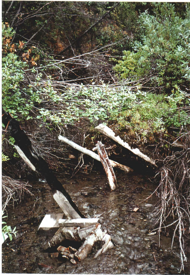
Photo 19. Adit seepage draining to French drain.
