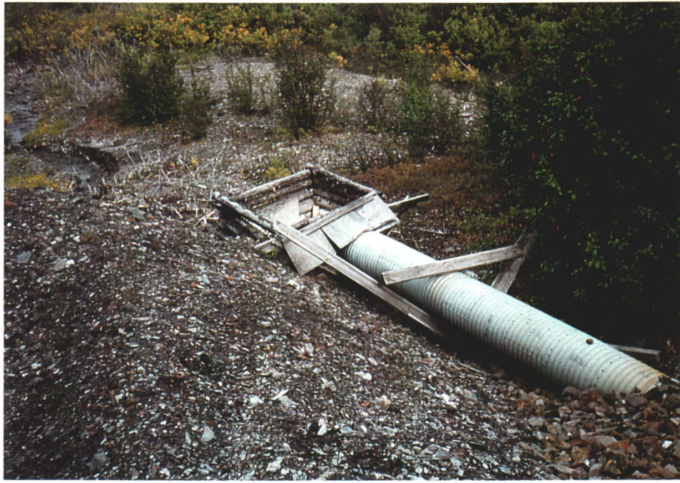
Photo 9. Furthest extension of French drain downslope 85 m from adit entrance.
