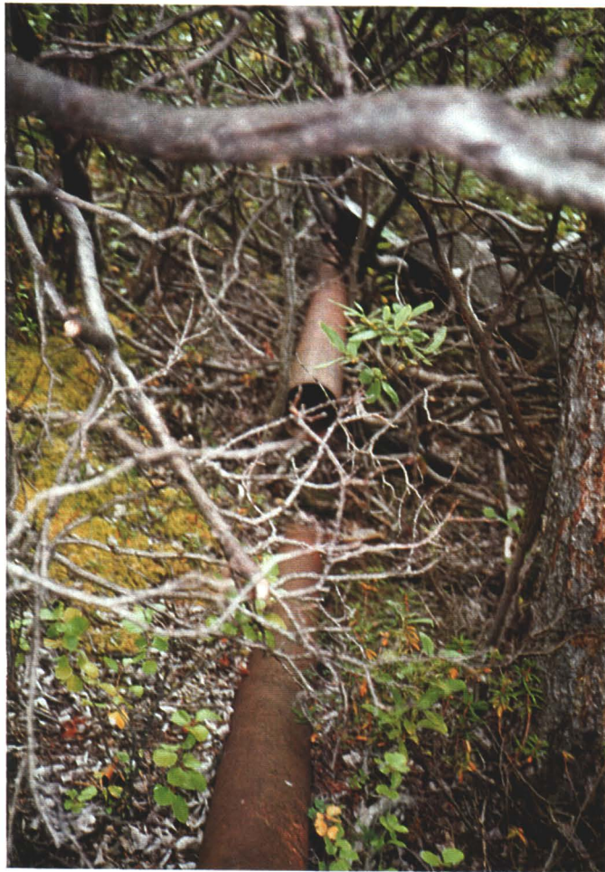
Photo 11. Pipe providing services to adjacent cabin.
