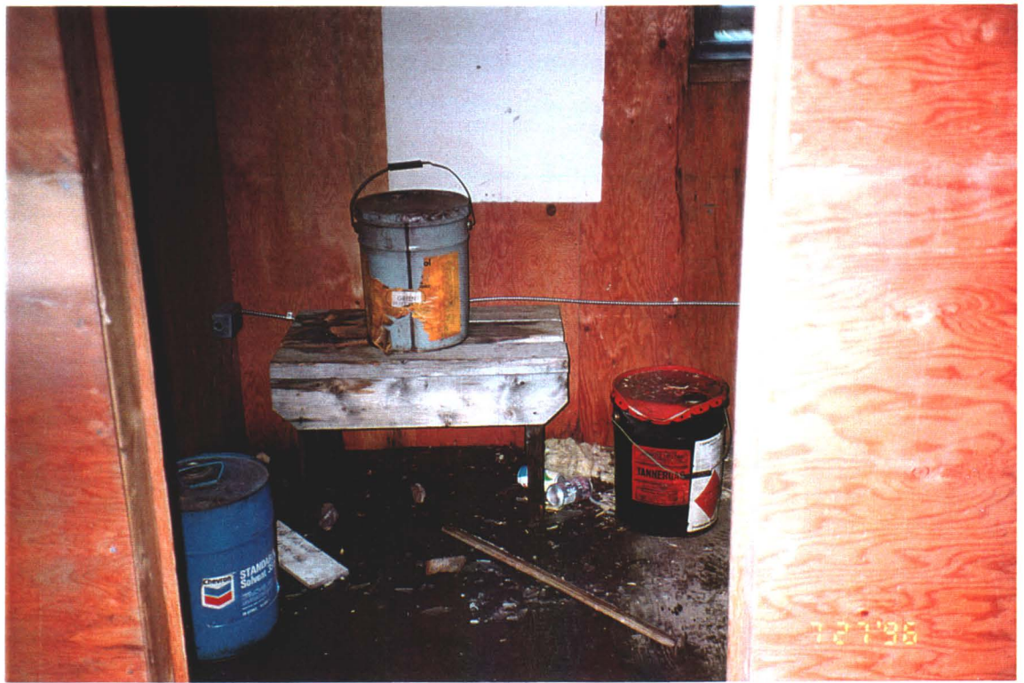
Photo # 41 - Three Pails containing Residual Contents located in a Storage Shed
