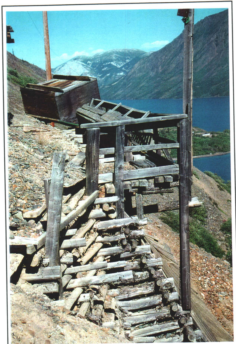
Photo # 23 - Retaining Wall and Toppled Shack
