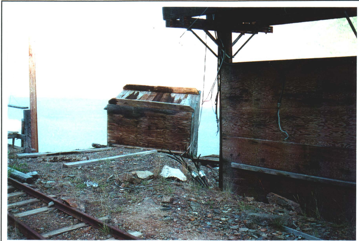
Photo # 20 - Shack on verge of toppling over Embankment
