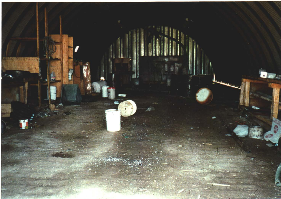
Photo 12. View of interior of maintenance shed. Note obvious signs of soil staining and waste oil containers (right rear).
