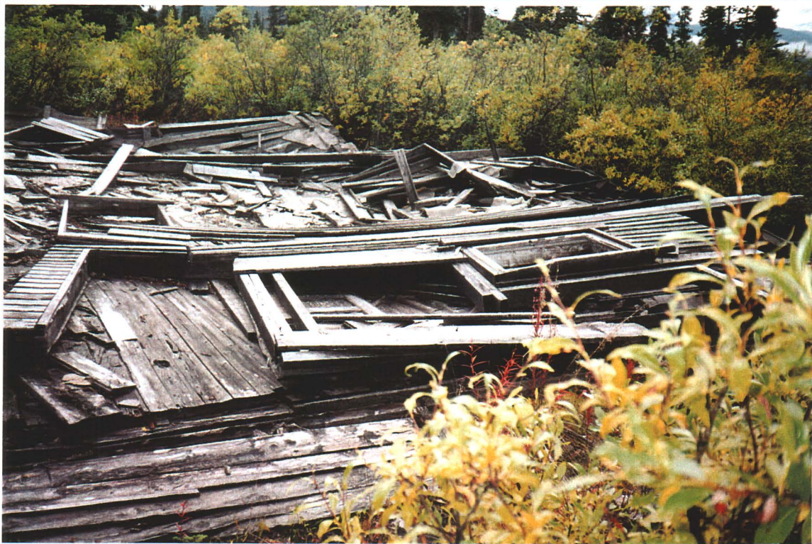
Collapsed building structure.
