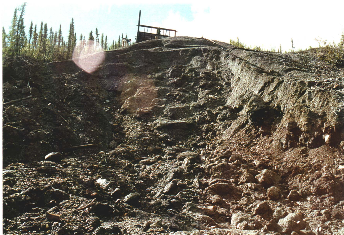
Photo 3. Slumped overburden and waste rock below crest of waste rock slope.
