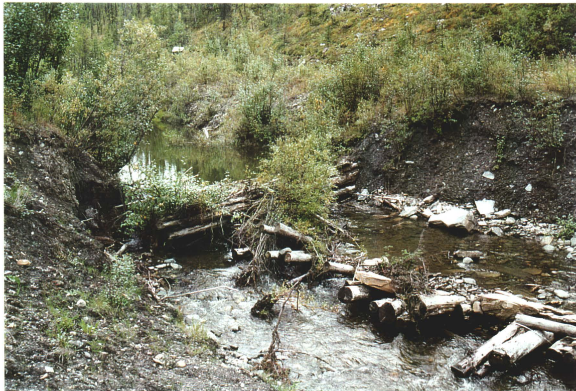
Photo 2. Collapsed bridge upstream from adit. Note ponded water behind cross-stream beams indicating partial flow blockage.
