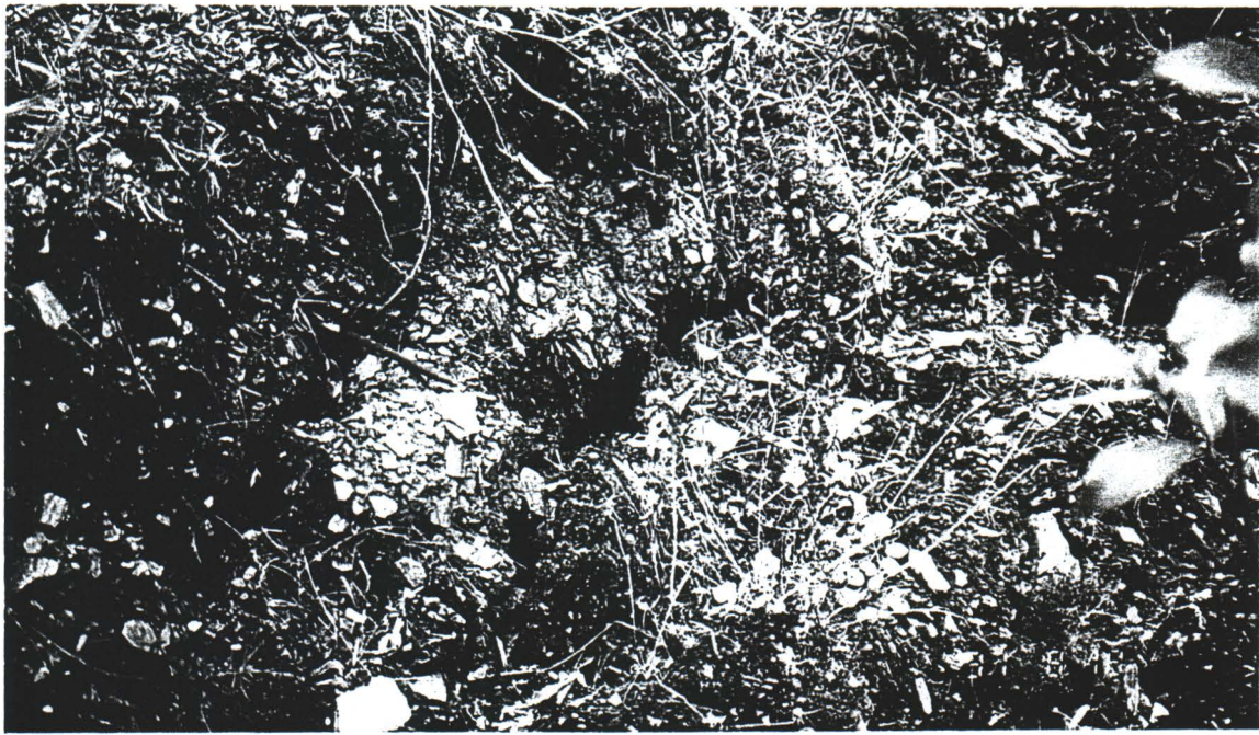
Photo #PA3: Evidence of slump failure along lower road. Movement due to eventual stabilization of loose fill material placed at excessive slope angles and without compactive effort.
