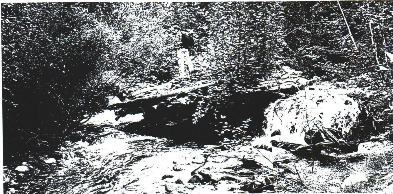
Photo #PA1: Bridge#1 collapsed into creek. Note log crib construction with earthen fill; note approximately 0.5 m drop in water level at right side of creek.
