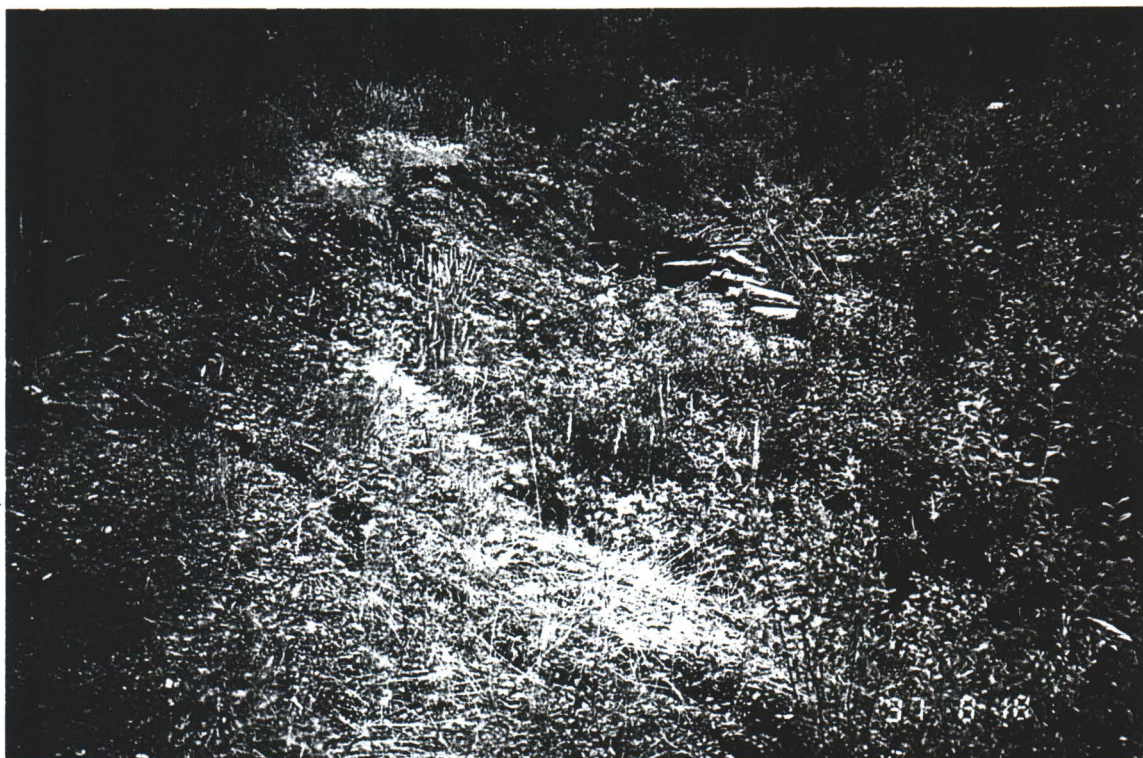
Photo #PA2: Note slump failures along north bank of creek just down stream of collapsed bridge #2.
