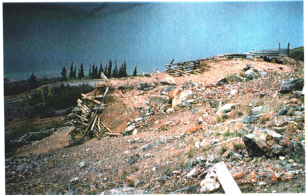
Photo #V4: Looking south east at lower retaining wall. Note sloughing of waste rock material; note poor condition of log cribbing supports.
