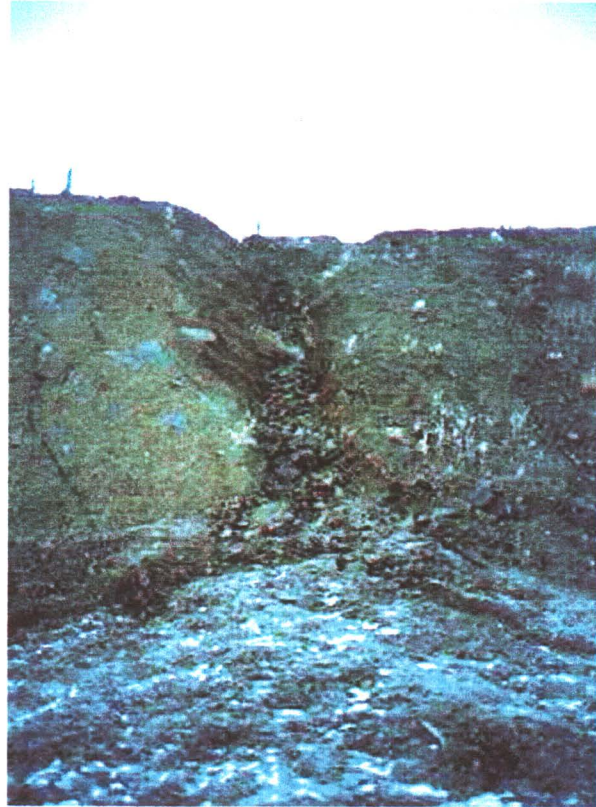
#19 Slope failure from seasonal run-off in waste rock dump at the La Forma Mine, October 1999.
