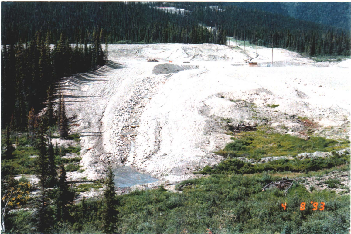
Photo 4 : General view of the reconstructed spillway chute at the Reclaim Pond dam.
