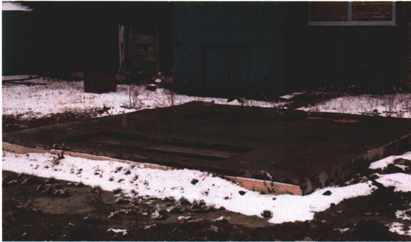
Photograph 6: Concrete pad on east side of main mill building (likely former location of main generator) with hazardous openings visible
