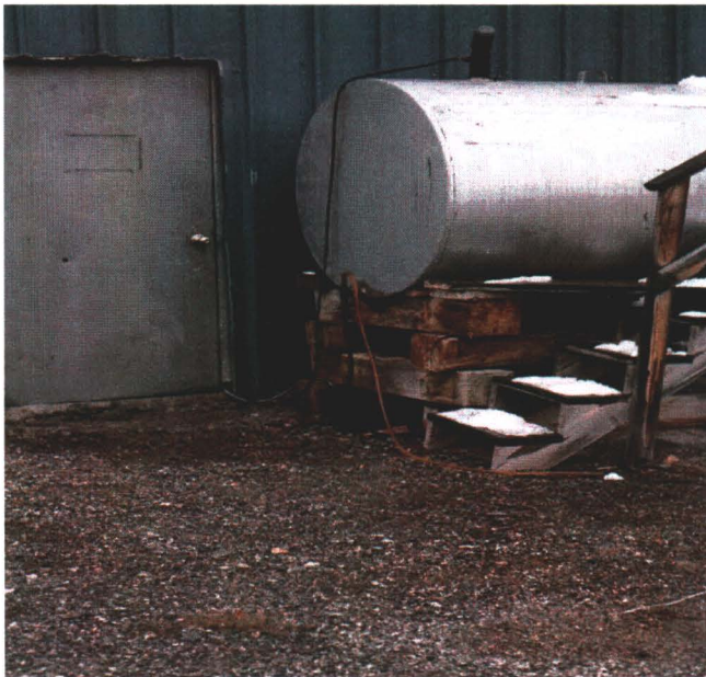
Photograph 7: Leaking diesel fuel AST (AST 1 in Figure 2) located near generator in maintenance building
