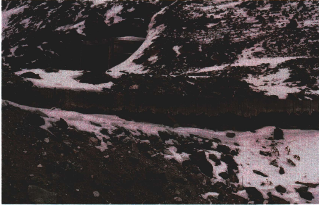
Photograph 20: Concrete slab which was placed on fill at lower portal and which has been undercut on both sides and poses risks of further undermining and a vertical drop
