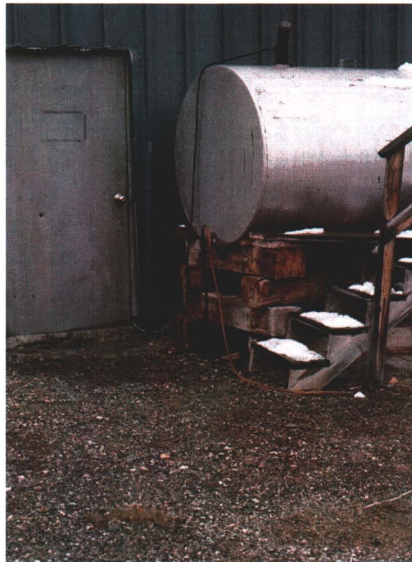
Photograph 3: Leaking diesel fuel tank for generator at rear of maintenance/core storage building (AST 1)
