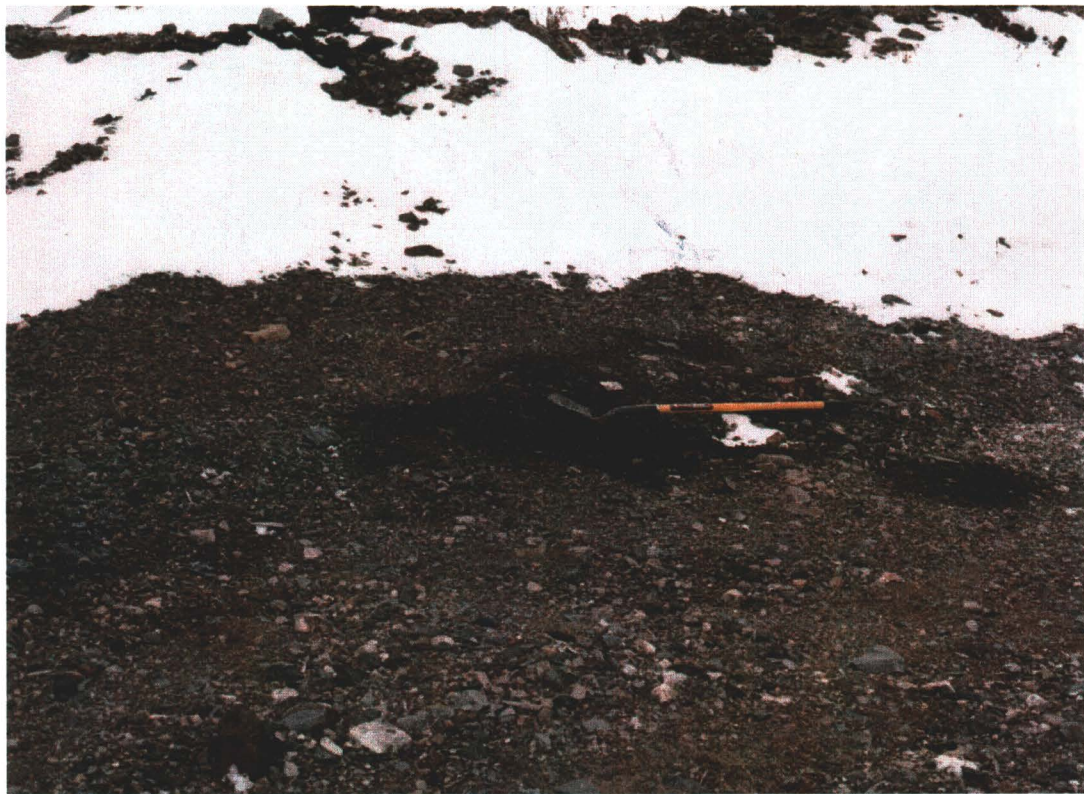
Photograph 21: Stained soil in the vicinity of the lower portal
