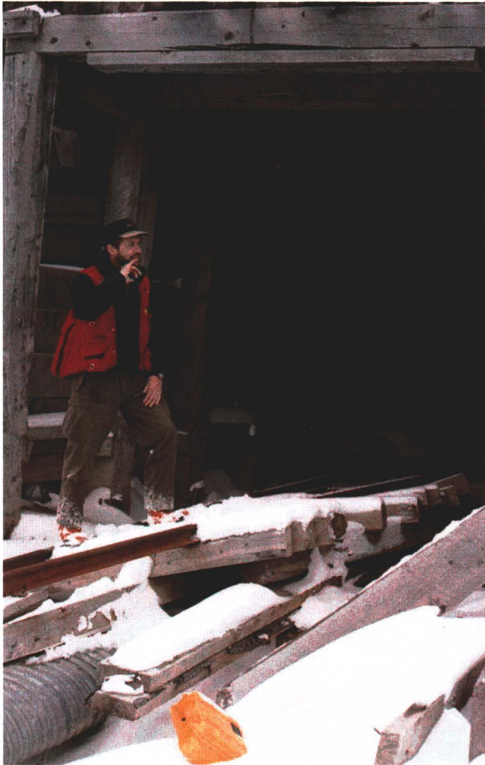
Photograph 15: Lower adit portal filled with ice (just beyond visible extent) and showing the destruction caused by earlier washout
