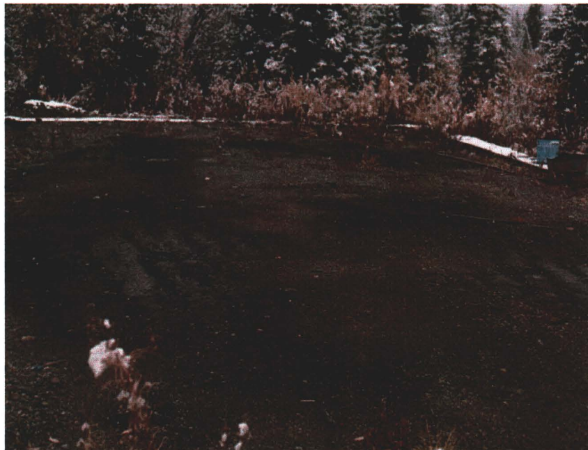
Photograph 12: View of floor of abandoned maintenance shed with darkest areas showing main zones of hydrocarbon contamination
