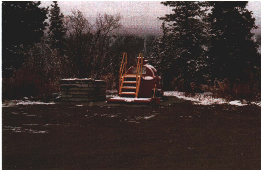
Photograph 8: Double walled AST (AST 2 in figure 2) located near mill
