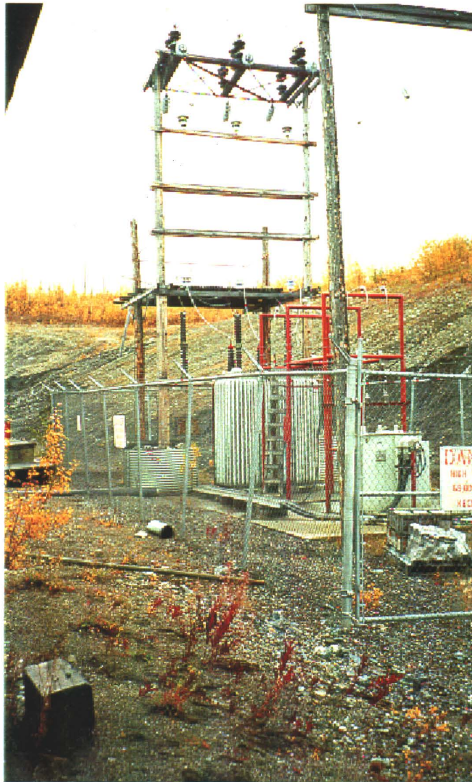
Photo 2-12: Power compound generating station.
