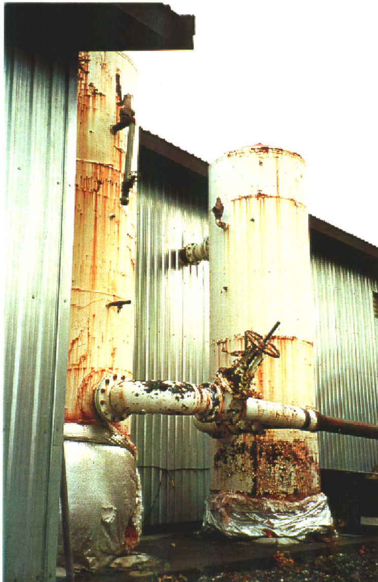
Photo 2-16: Air compressor tanks, south wall.
