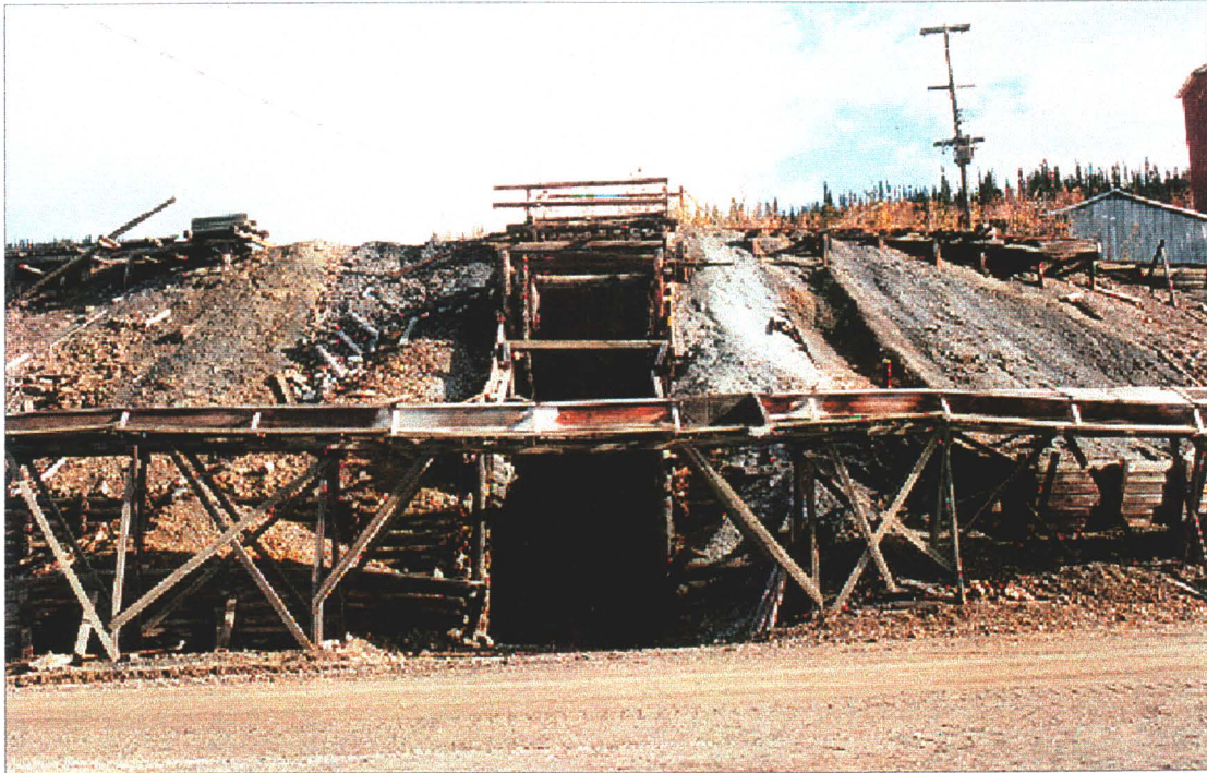
Photo 3-3 : Elsa Mine. Elsa 400 ore chute and grizzly from below. Looking southeast. Note steep banks of waste rock.
