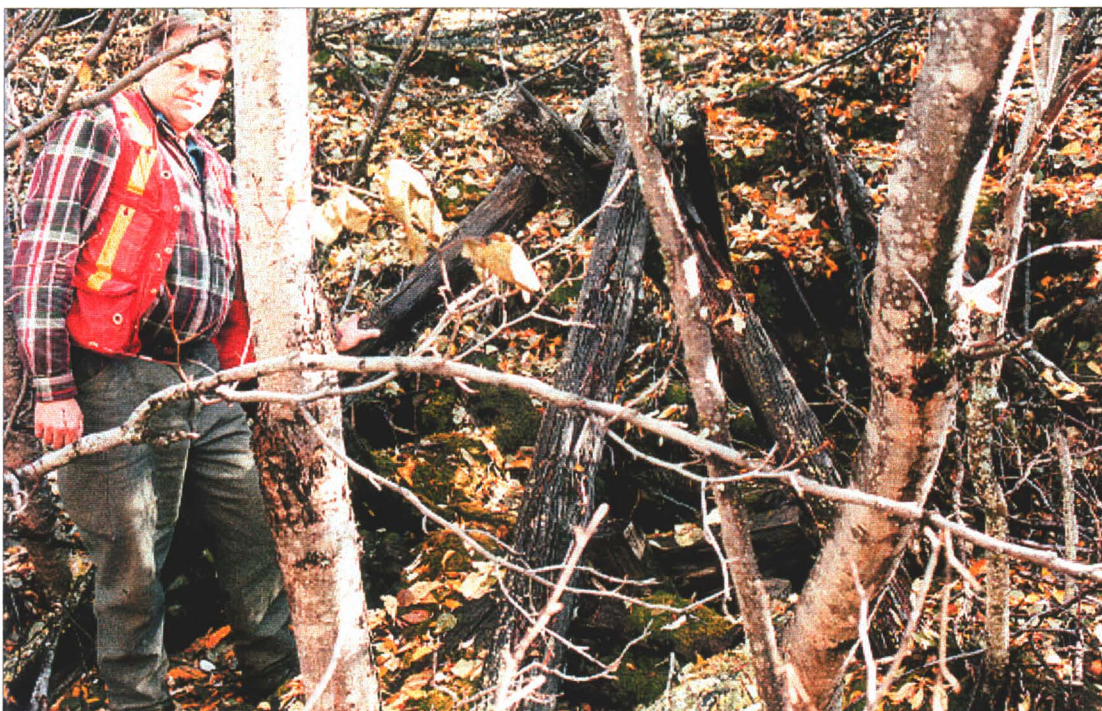
Photo 3-10 : Elsa Mine. Tick shaft. Rotting timberframe, collapsed adit. Looking south.
