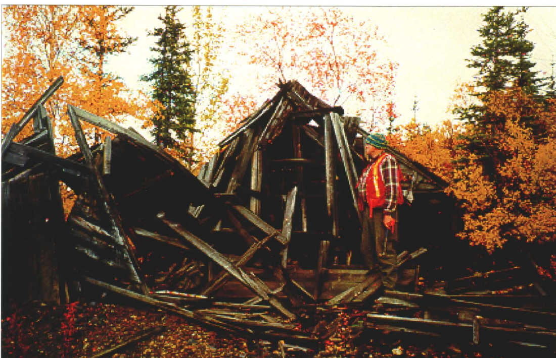
Photo 4-2: Collapsed structure above raise. The raise is located at the intersection of the powerline and roadway approximately 500m above the main Dixie site. (Azimuth 95°)
