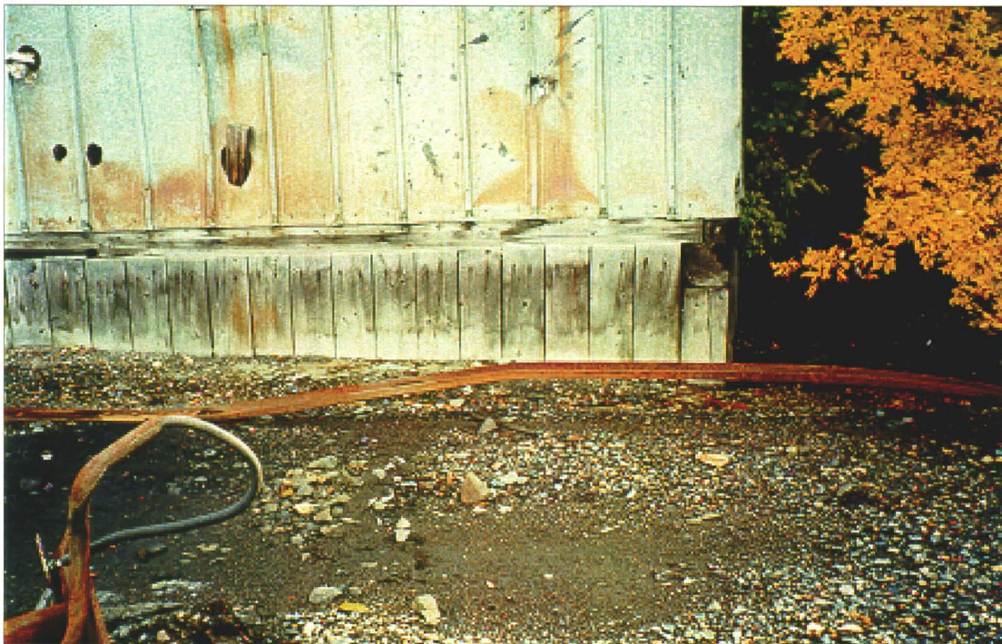
Photo 4-8: Stained soil on the west side of building 4A. (Azimuth 135°)
