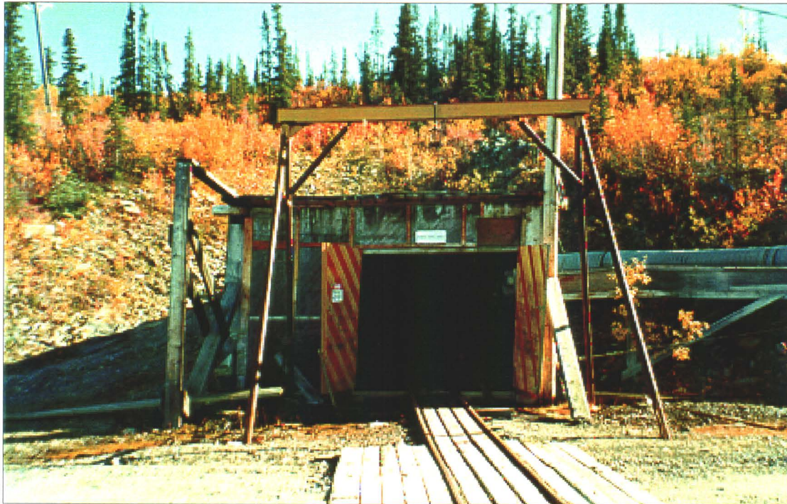
Photo 6-15 : Ruby 400. Adit structure with rail tracks extending from the structure and utilidor on right..
