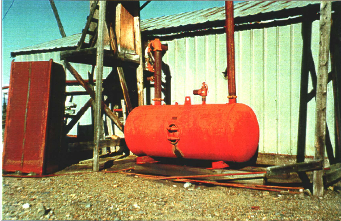
Photo 6-20 : Ruby 400. Receiving tank located on the exterior wall of the boiler house.
