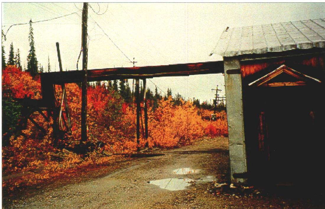
Photo 6-14 : Ruby 400. Utildor from adit structure to garage. Transformer compound is in the background.
