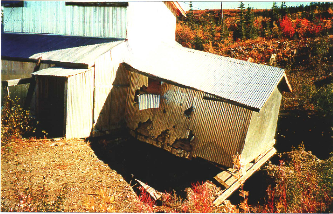
Photo 6-2 : Ruby Shaft. South portion of shaft house over opening has collapsed.
