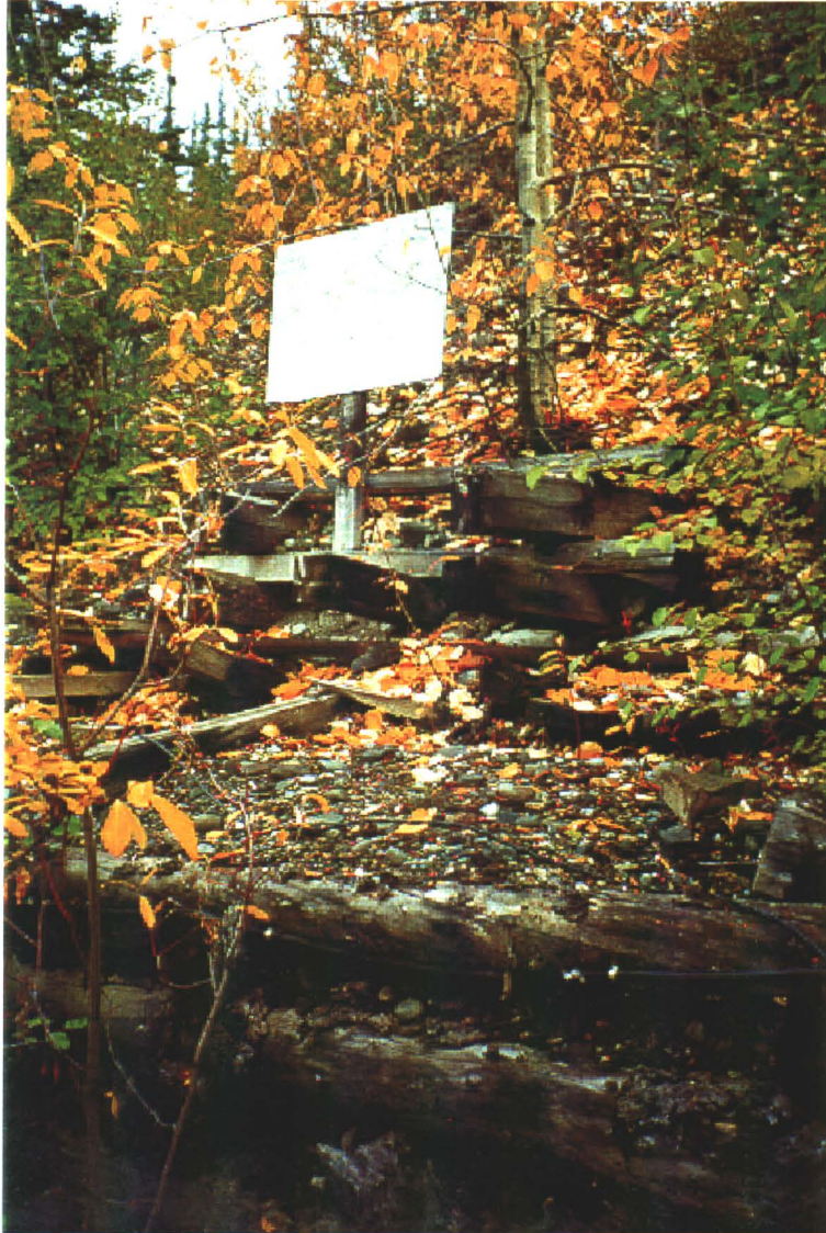
Photo 7-13: Old adit structure that has collapsed and caved in.
