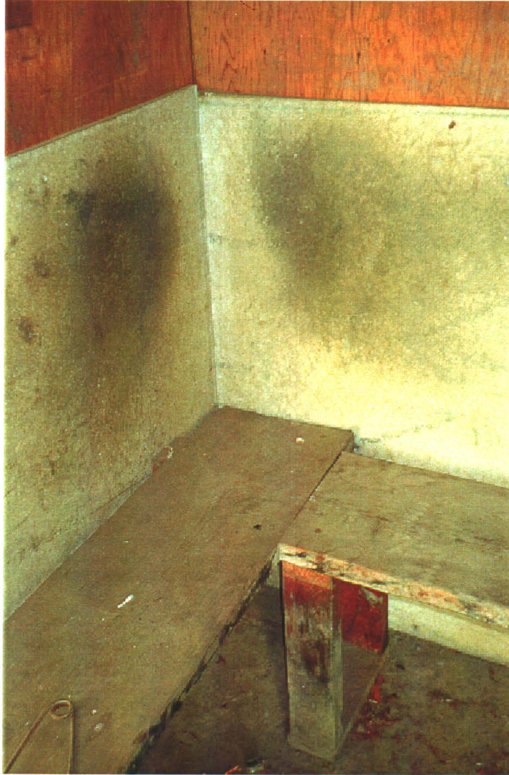
Photo 7-9: Interior of the lunchroom. Note the asbestos board on the walls.
