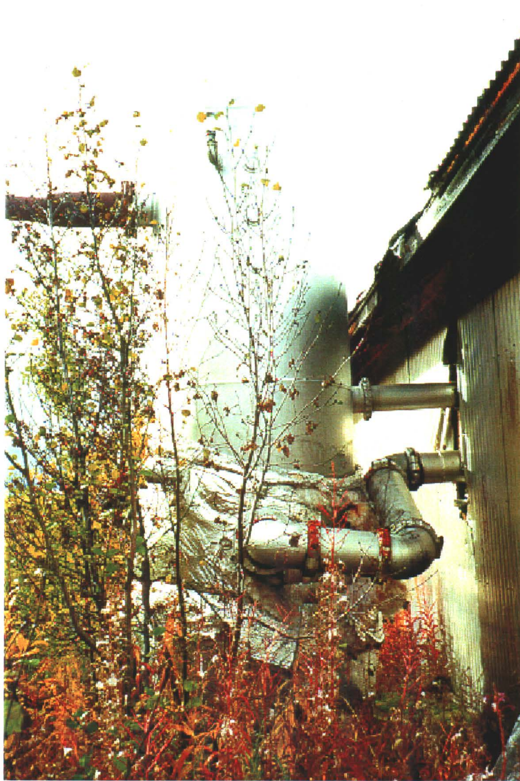
Photo 7-5: Receiving tank located on the outside of the garage structure. Tank was insulated with fibreglass.
