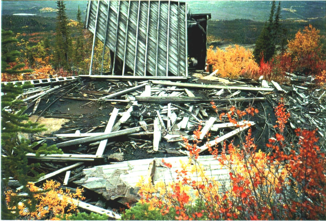
Photo 9-11. Concrete foundation of storage tank with debris from storage tank. Building in the background.
