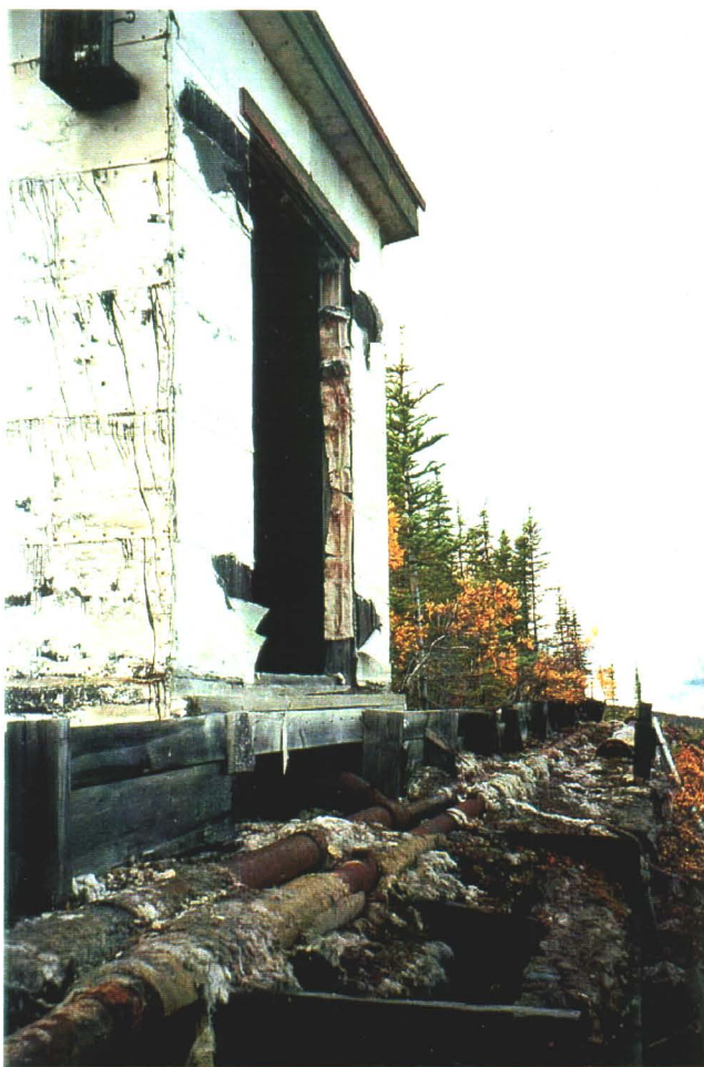
Photo 9-8. Building 9B. Note wooden construction and tar paper siding. Also note metal piping and remnants of insulation that comprises the utilidors.
