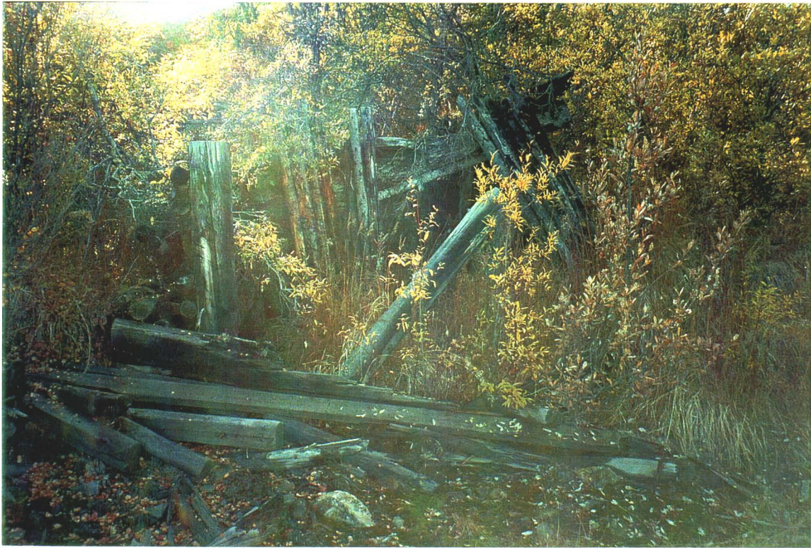
Photo 11-5. Galkeno 200 level adit. Portal is open but is unsafe. The timbers of the portal are collapsing.
