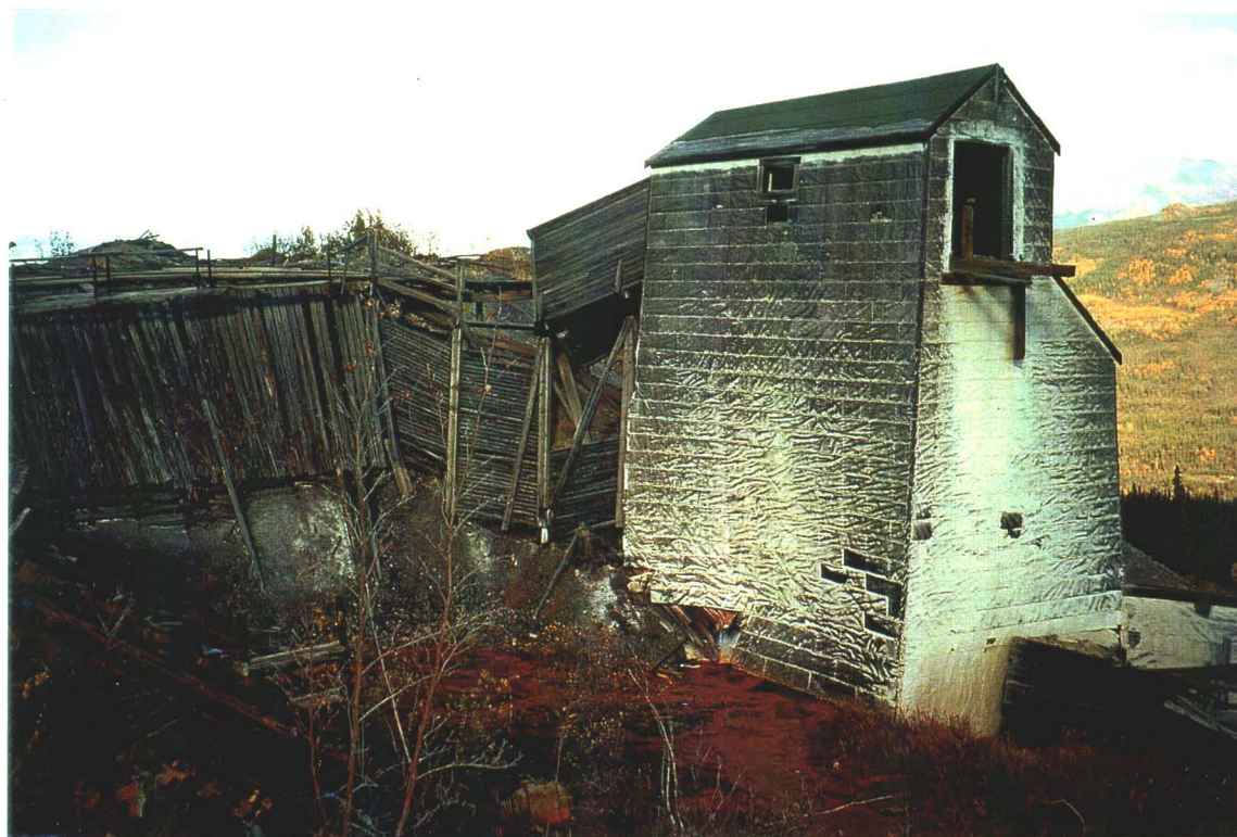
Photo 11-12. Building 11B - Loading Elevator, looking northwest. The building is located on the waste rock dump outside the 300 level adit. Note how the building is leaning away from the waste dump (also see Photo 11-14).
