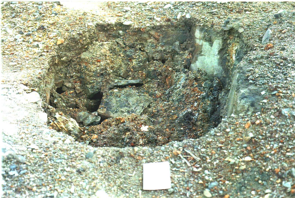
Photo 11-2. Subsidence over adit workings, near the McLeod Shaft. The collapsed area measures approximately one meter across.
