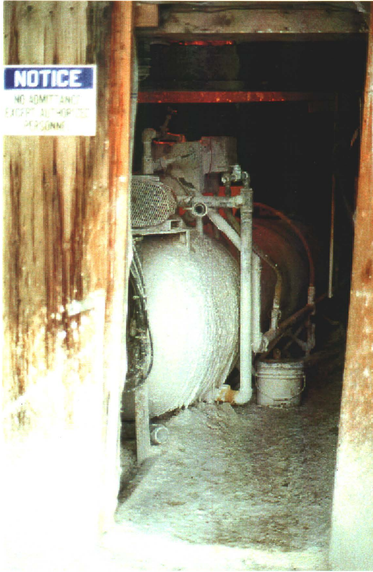
Photo 12-4: Water treatment facility within the portal. (Azimuth 270°)
