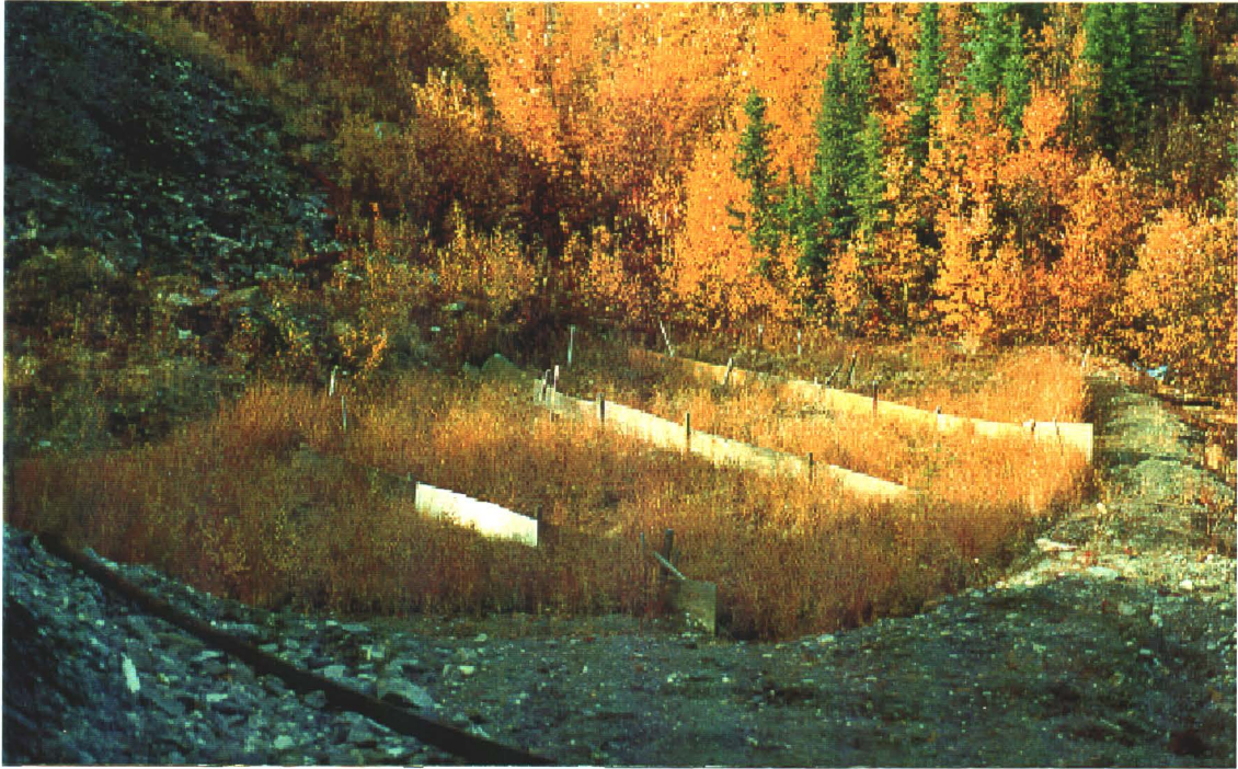
Photo 12-7: Constructed wetland plot with wooden baffles. (Azimuth 345°)
