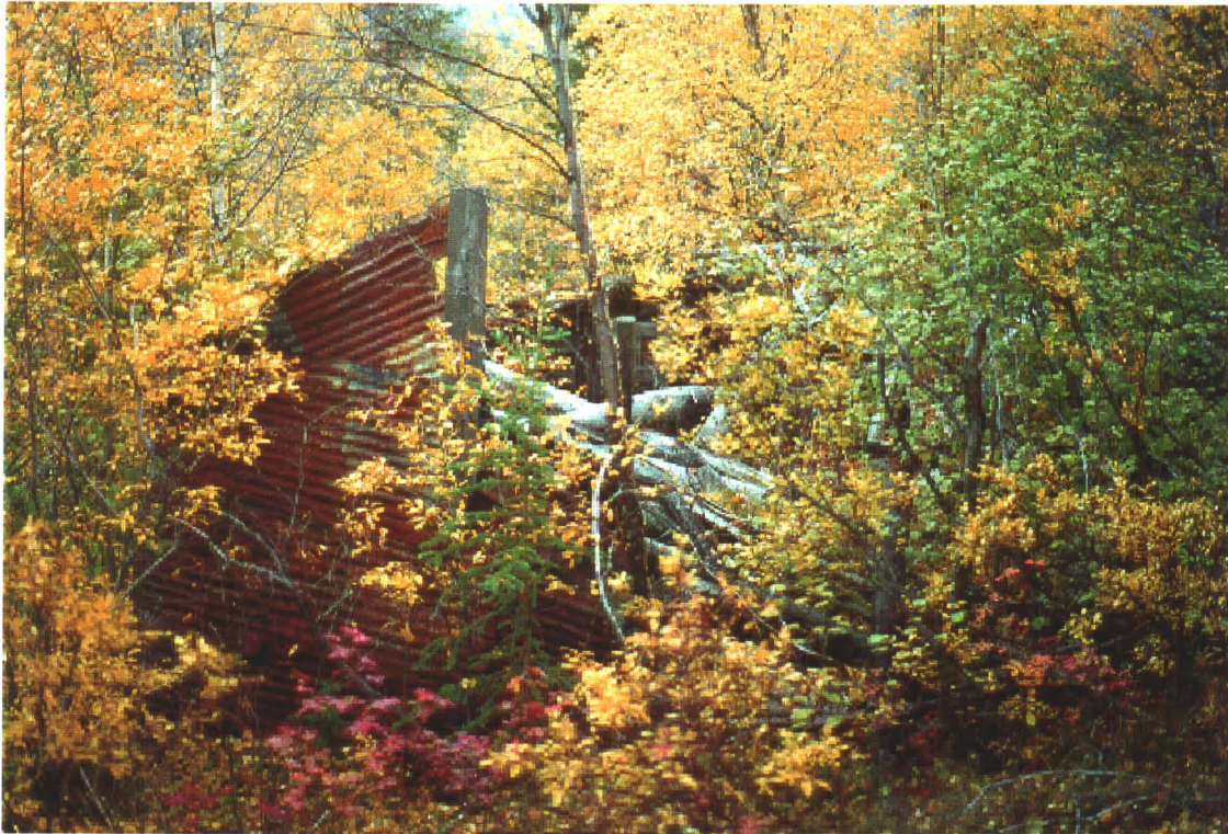
Photo 16-3: Collapsed log cabin with metal sheeting which covers the north side of the cabin. (Azimuth 150°)
