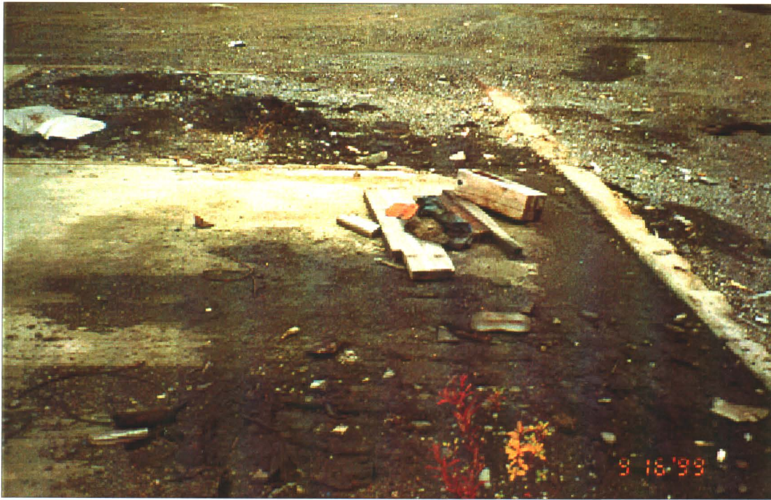
Photo 19-20: Extensive staining in sumps at building 19G.
