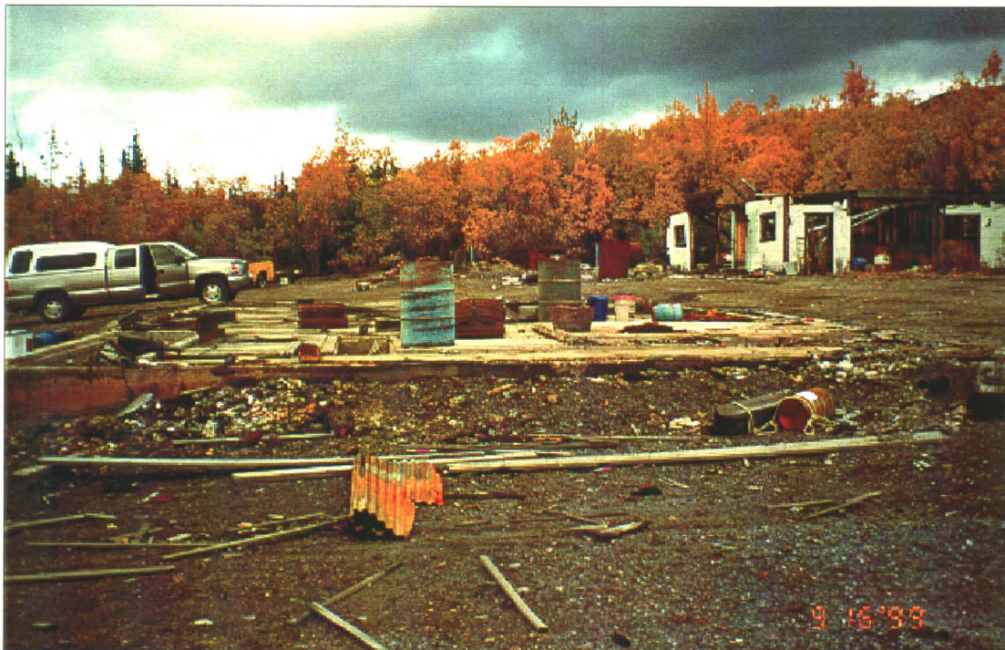
Photo 19-11: Concrete foundation (building 19G) and much debris.
