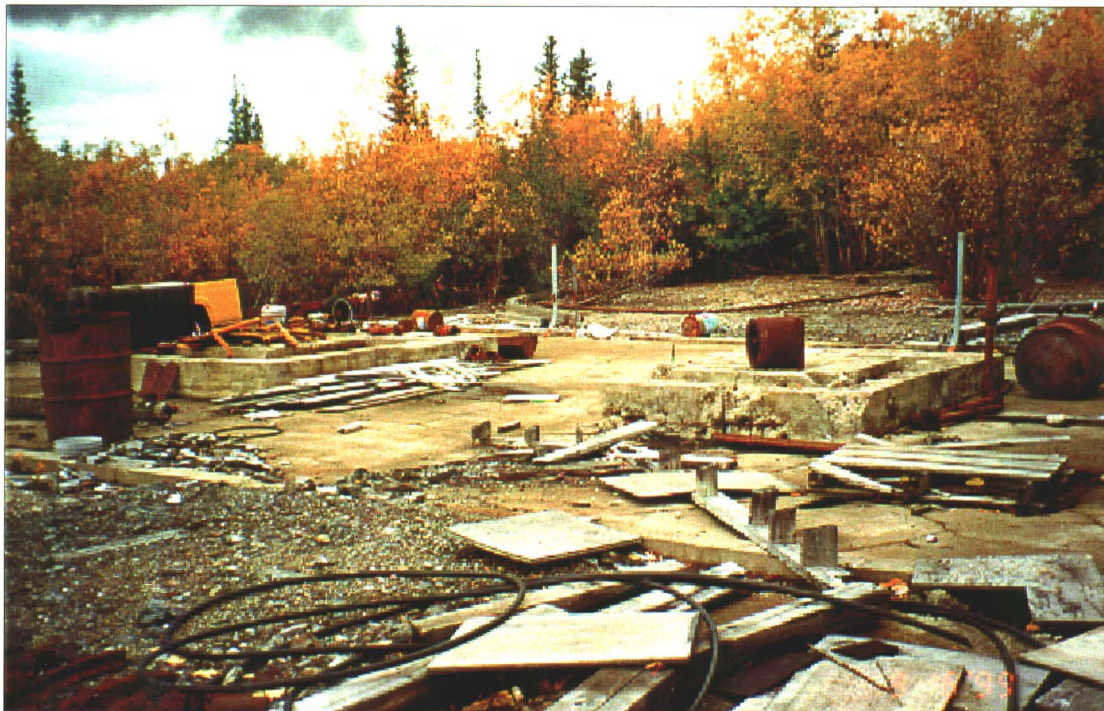
Photo 19-10: Concrete foundation (building 19F) with much metal and debris.
