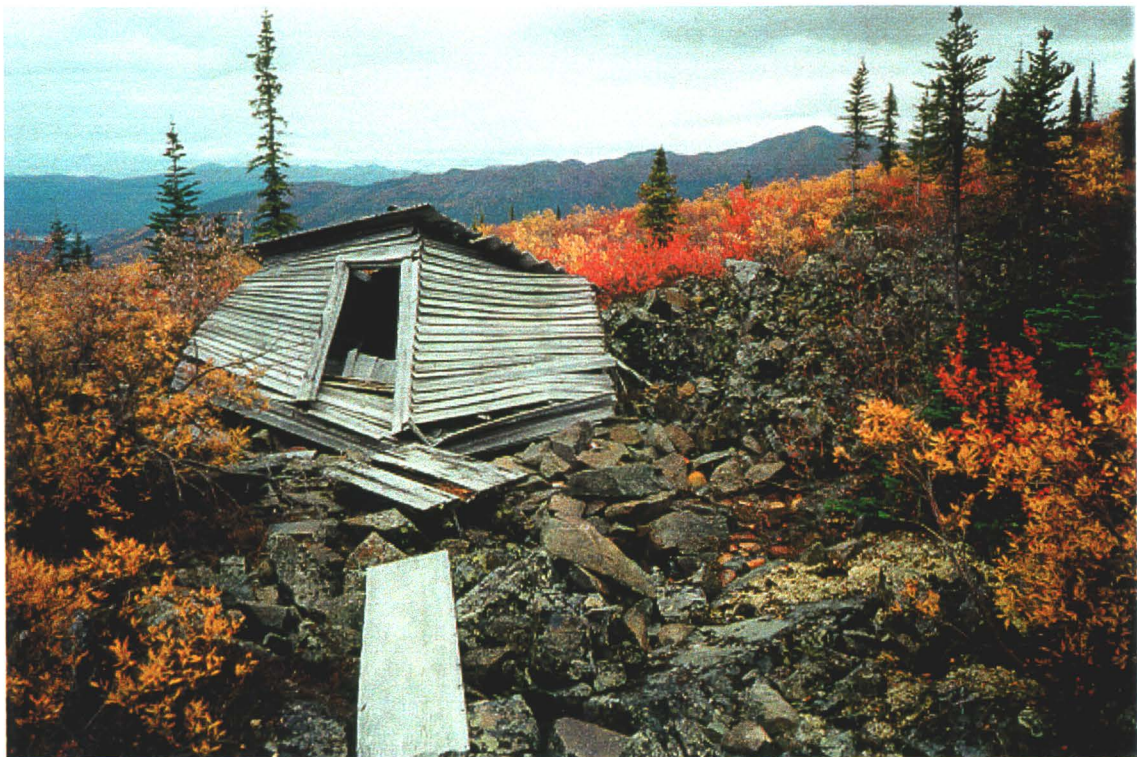
Photo 21-13: Collapsed shed (Bldg. 21-E) (Azimuth 000°)
