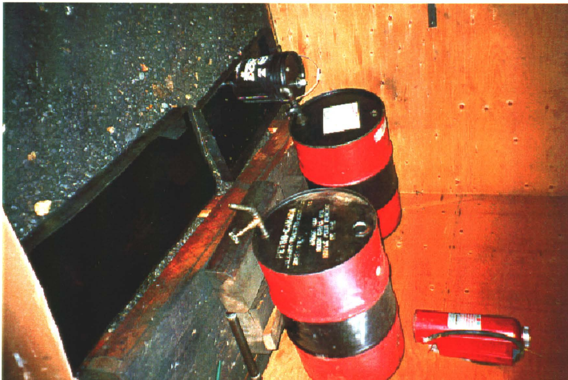
Photo 22-6: Oil barrels fitted with dispensing valves located inside compressor house. Spill trays are filled with oil and hydrocarbon staining is evident on floor.
