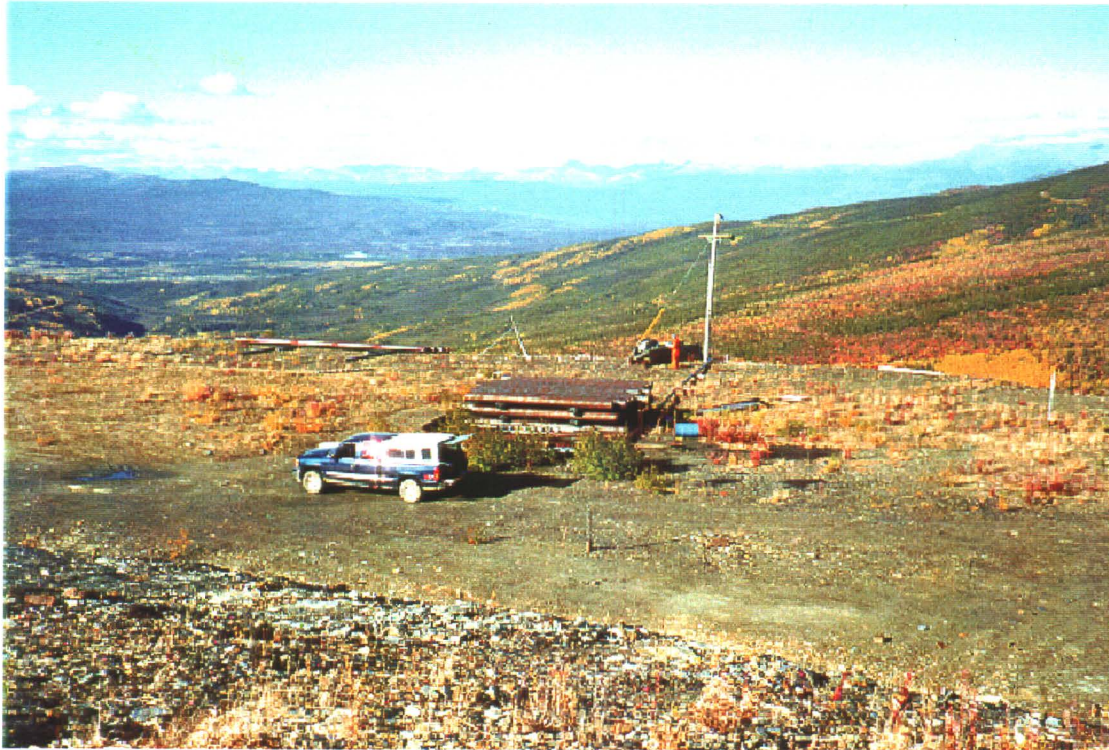
Photo 22-13: Bellekeno Backfill site. Drilling site is at centre of photograph next to laydown of pipes.
