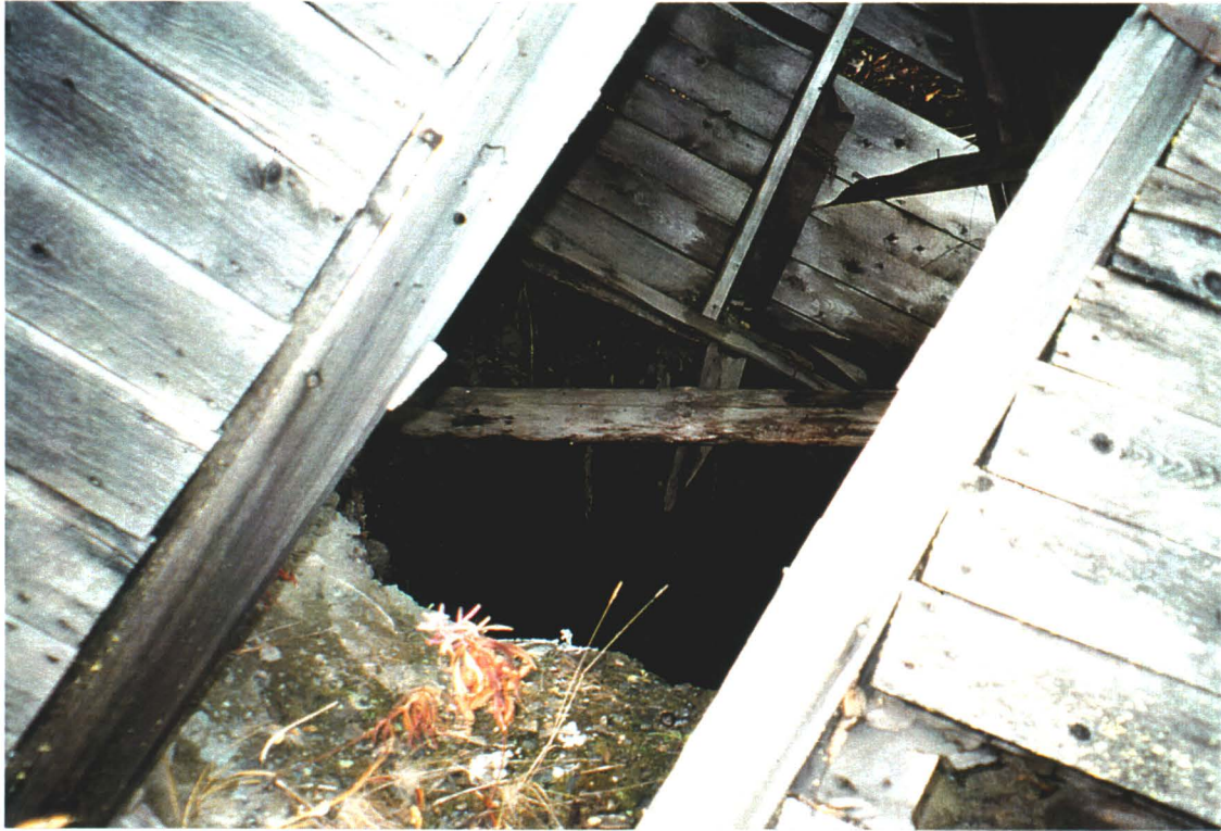
Photo 22-11: Collapsed structure enclosing shaft across Sourdough Hill Road from Bellekeno 100 level adit
