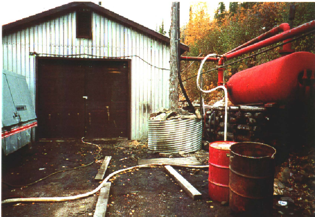
Photo 22-4: Compressor house at Bellekeno 625 level adit (Building 22C). Hydrocarbon staining is evident at entrance.
