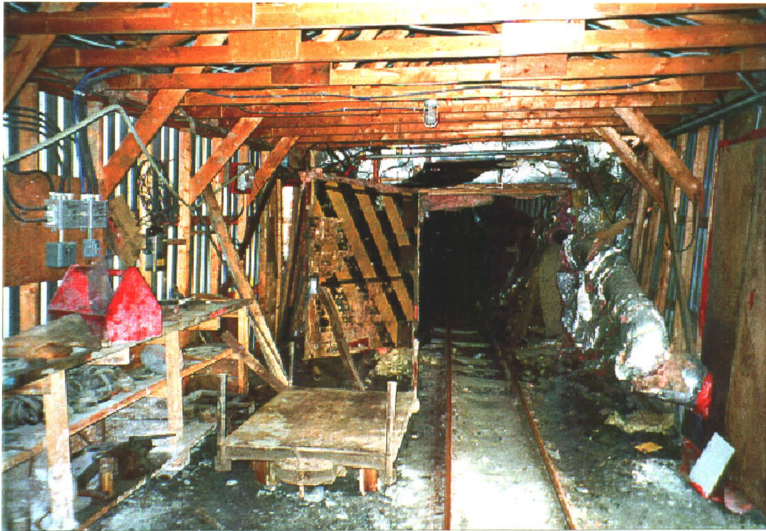
Photo 22-3: View of Bellekeno 625 level adit from inside of adit building (Building 22A)
