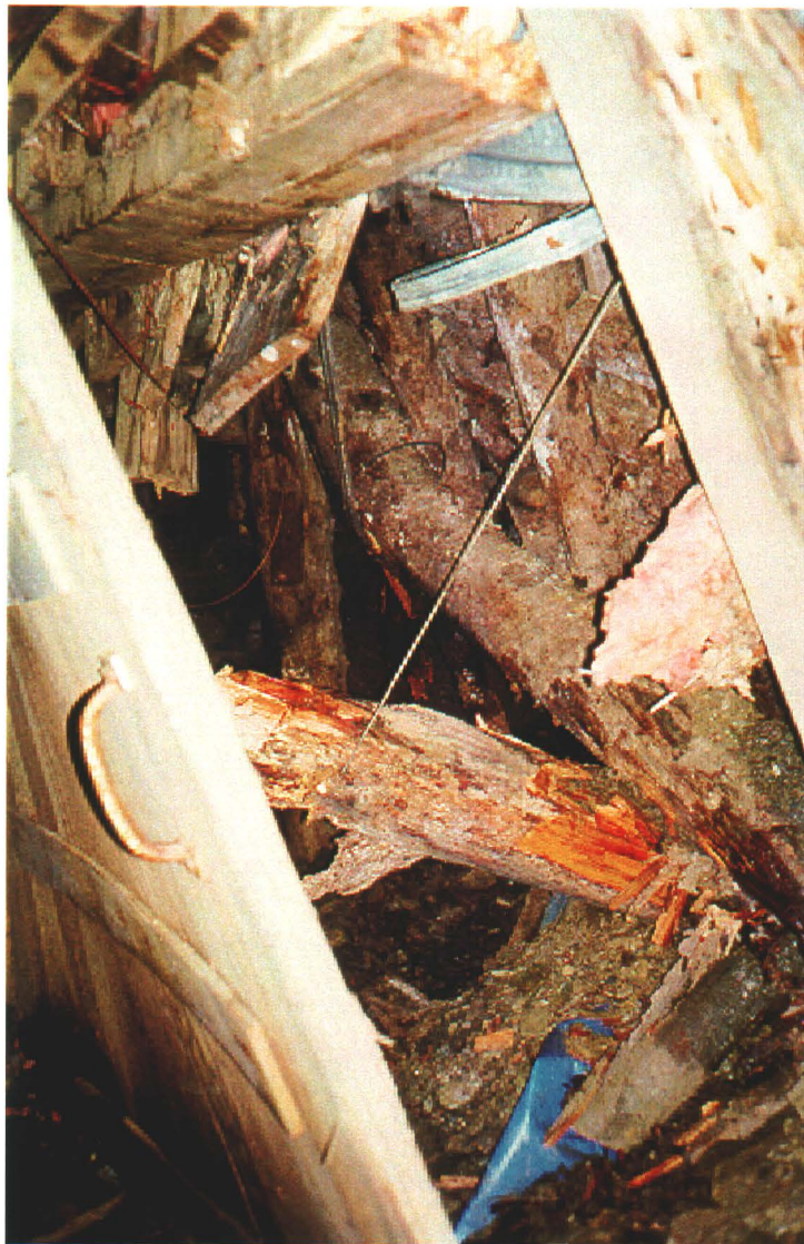
Photo 25-9: Collapsed portal timbers behind door.
