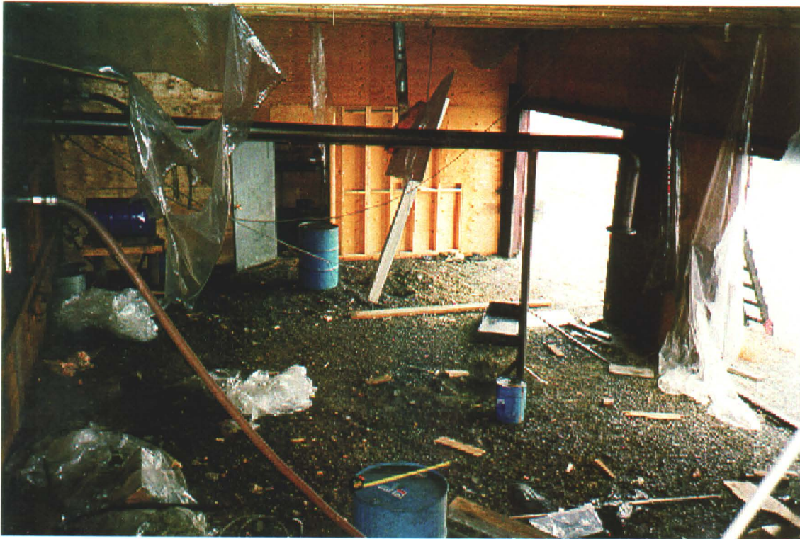
Photo 25-15: Interior of workshop bays. Note drum of transmission oil and pails of waste oil in left corner. Test pits located just right of far up-right drum (TP01) and blue pail of solvent near centre (Tp02). Workshop area through door on far wall. (Azimuth 180°)
