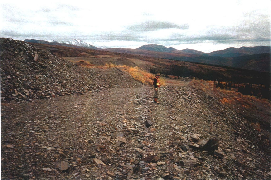
Photo 25-12: Tension cracks on edge of waste rock pile. Note slumped edge running along edge to mapper. (Azimuth 180°)
