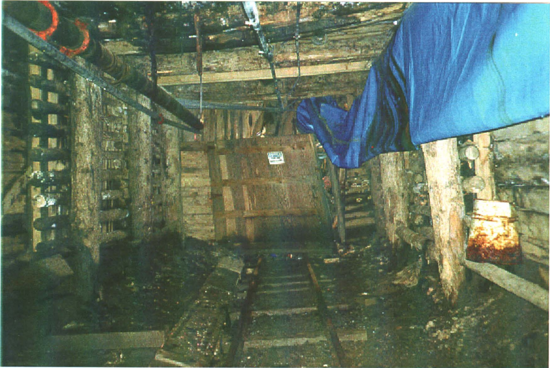
Photo 25-8: Interior of portal. Note drainage ditch to bottom left and partially collapsed door. (Azimuth 060°)
