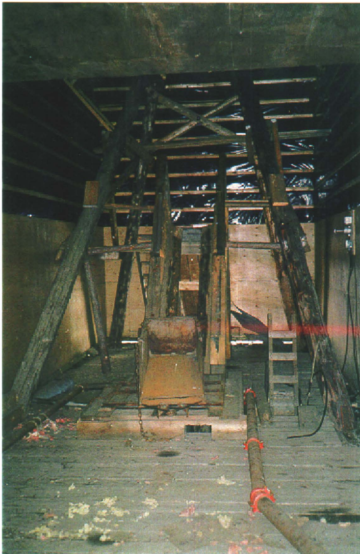
Photo 26-7: Interior of Lucky Queen headframe building (Bldg. 26-A) showing open manway and boarded shaft opening.
