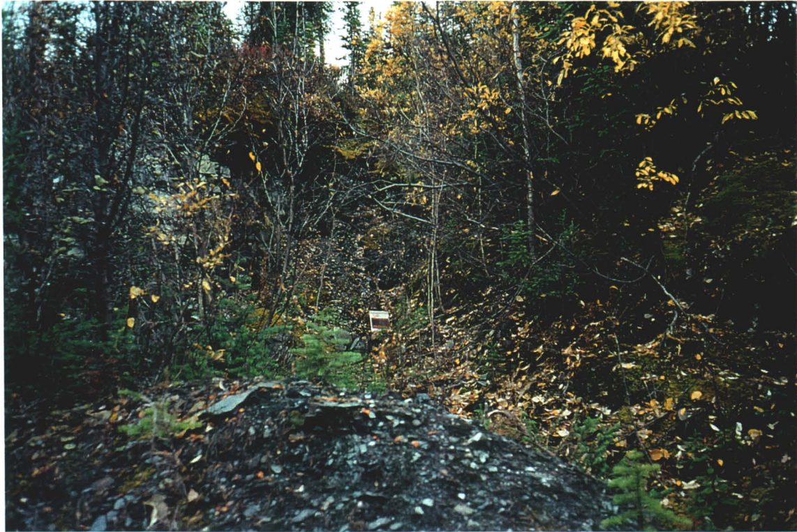
Photo 27-3: Collapsed adit portal (A02). (Azimuth 220°)
