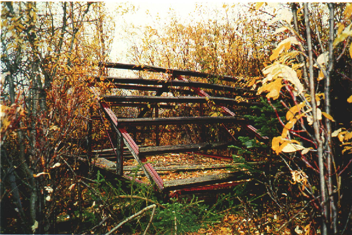
Photo 27-6: Collapsed steel building frame (Bldg. 27-2). (Azimuth 120°)
