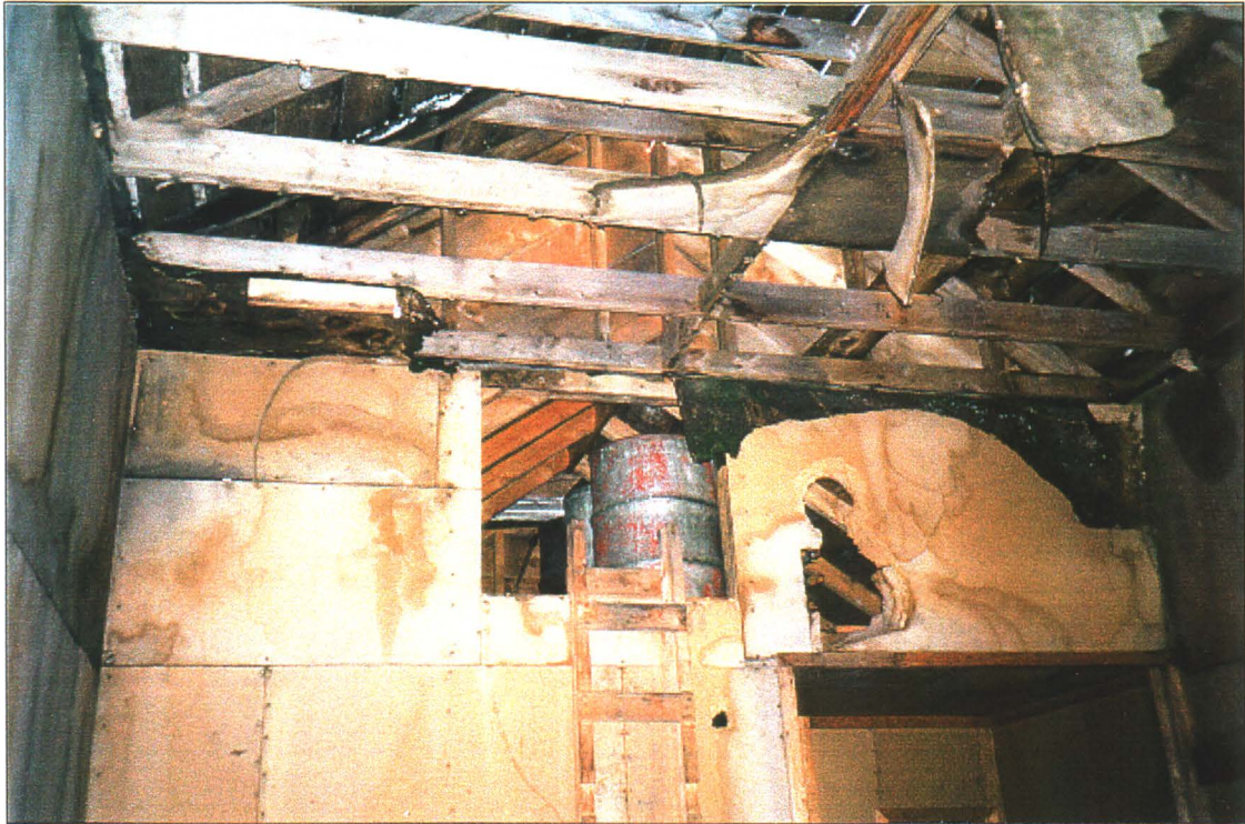
Photo 31-7: Interior of dry (Bldg 31-A) showing rafters, wallboard and water tanks for shower and sauna.
