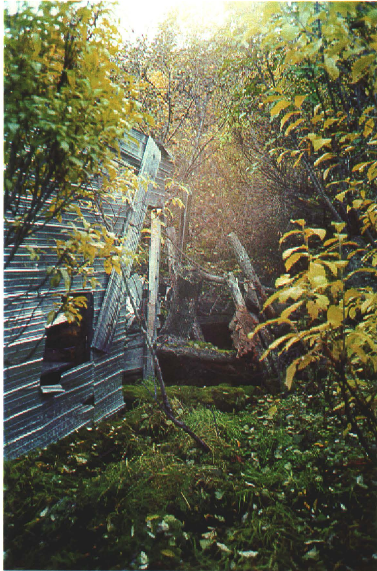
Photo 31-4: Collapsed middle adit portal and storage shed (Bldg. 31-B). Note damp ground from mine seepage. (Azimuth 160°)
