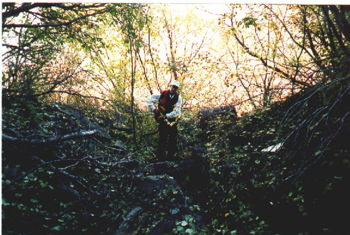
Photo 31-6: Collapsed lower adit portal. Photo Direction (Azimuth 032°)
