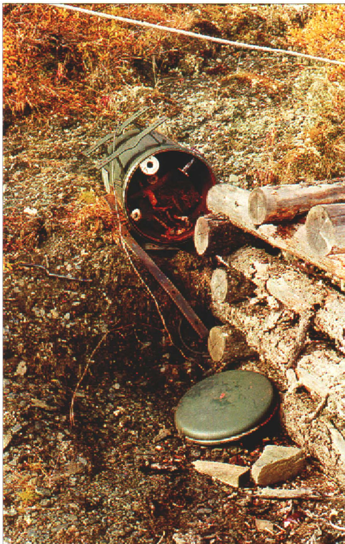
Photo 32-26 : Keno 200. Fallen capacitor / transformer by tower.
