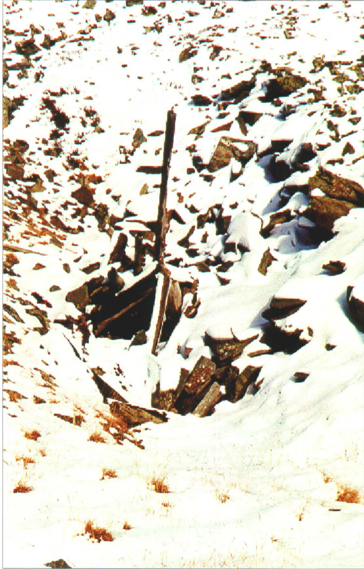
Photo 36-1 : Keno No.9 Collapsed log timbers mark the location of the No.5-2 Vein Adit. (Azimuth 025°)
