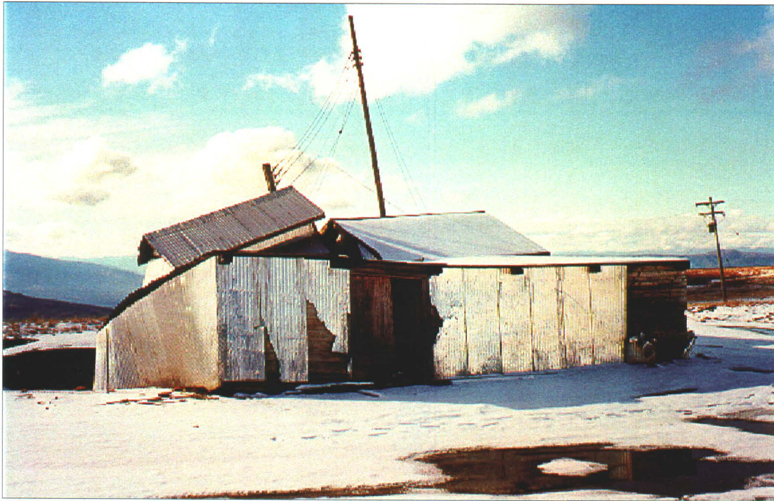
Photo 36-2 : Keno No.9 Shamrock J18 Vein Raise Building (36-A). Note collapse of building into failing underground workings and fencing around opening. Also, transformer on power pole in background. (Azimuth 290o ).
