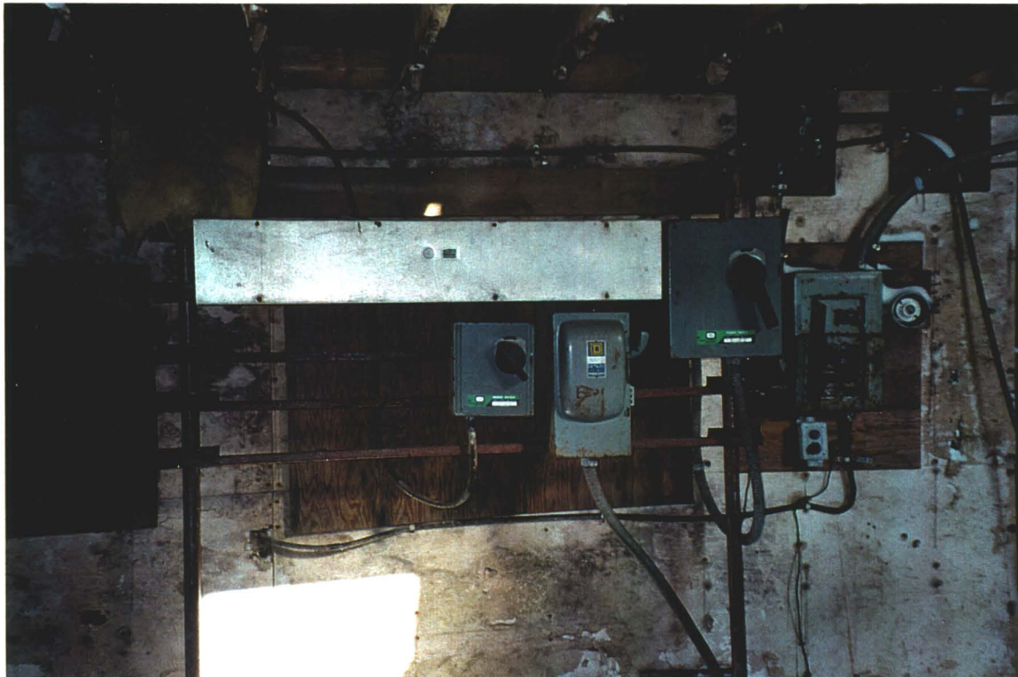
Photo 36-8: Keno No. 9 Electrical panel inside Building 36A.
