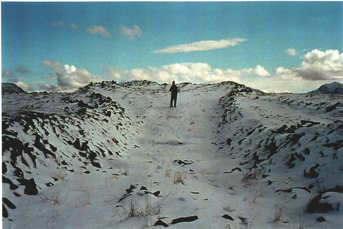
Photo 36-7 : Keno No.9 View of Trench L5 located on the No.4 vein. (Azimuth130°)
