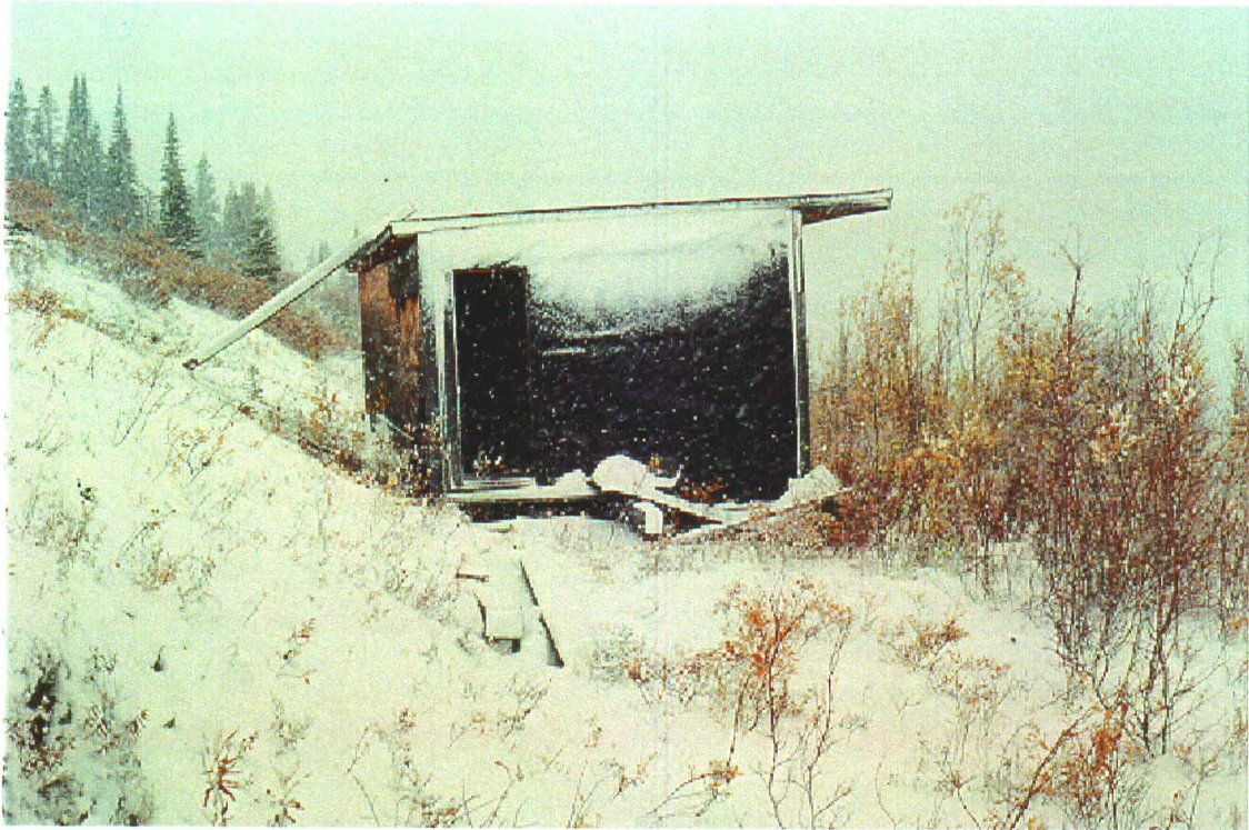
Photo 50-6: Building 50A with a small pile of wood debris out front (Azimuth 270°)
