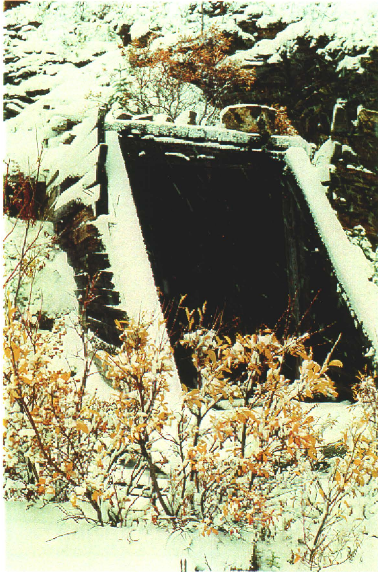
Photo 50-1: The large wooden structure is the portal to the Homestake adit. (Azimuth 225°)
