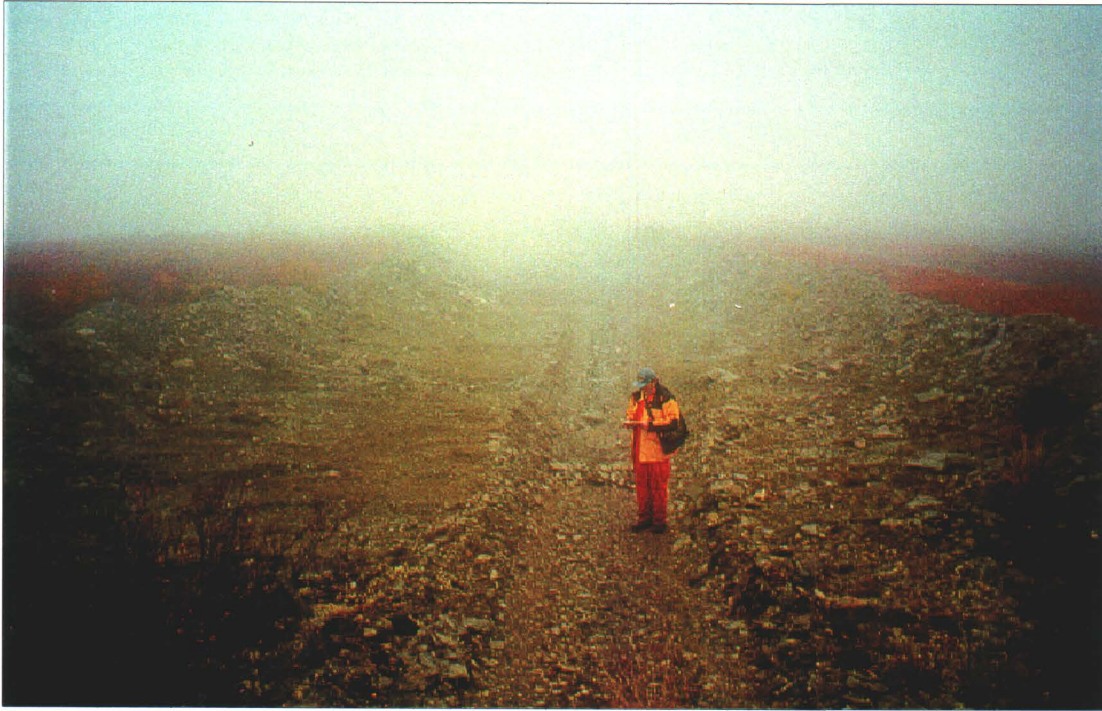
Photo 52-7: View along length of large trench (Trench 1) located 2 km south of Windy and Casy workings on Bob claim. (AZ 138°)
