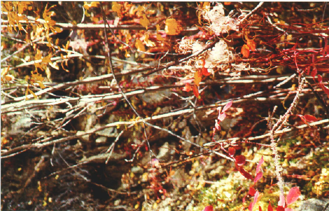
Photo 54-2: Obscured view of collapsed adit (Adit 1) at Hogan site.
