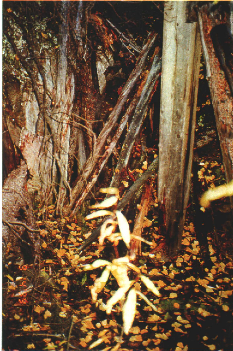
Photo 61-1: Timbers partially obscuring entrance to collapsed adit.
