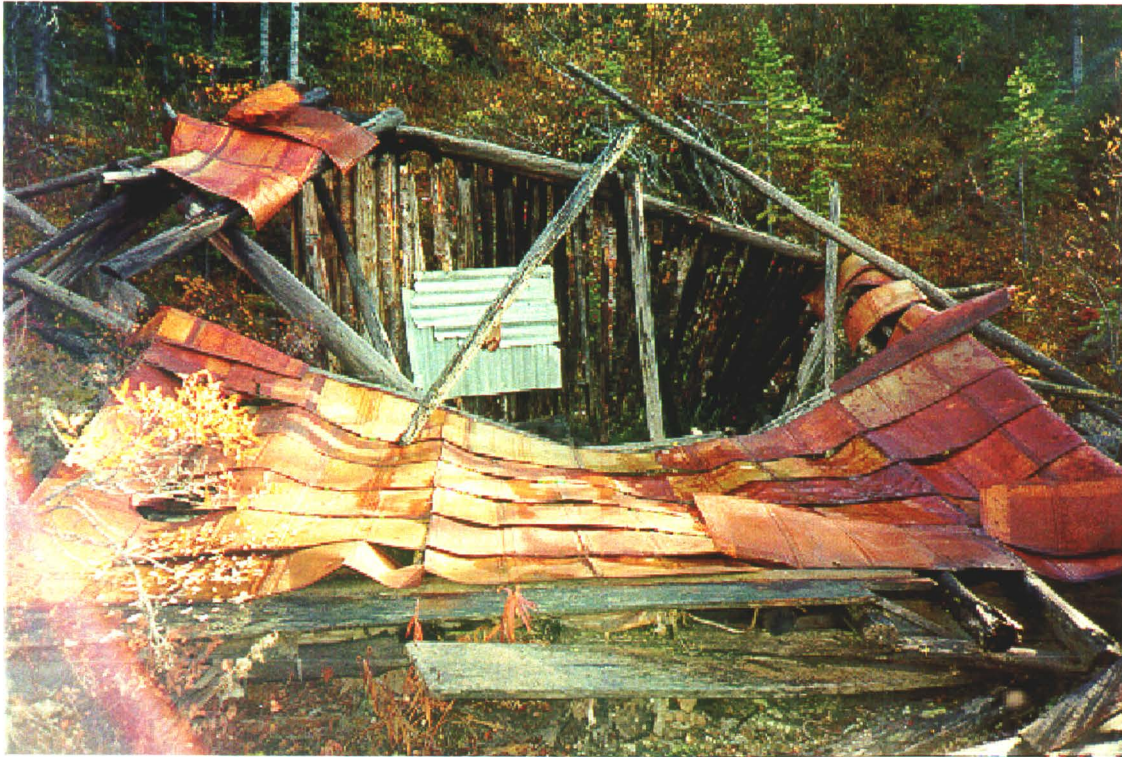
Photo 71-1: Collapsed shed building (Bldg. 71-2) over shaft A02. Note pulley on cross beam. (Azimuth 140°)
