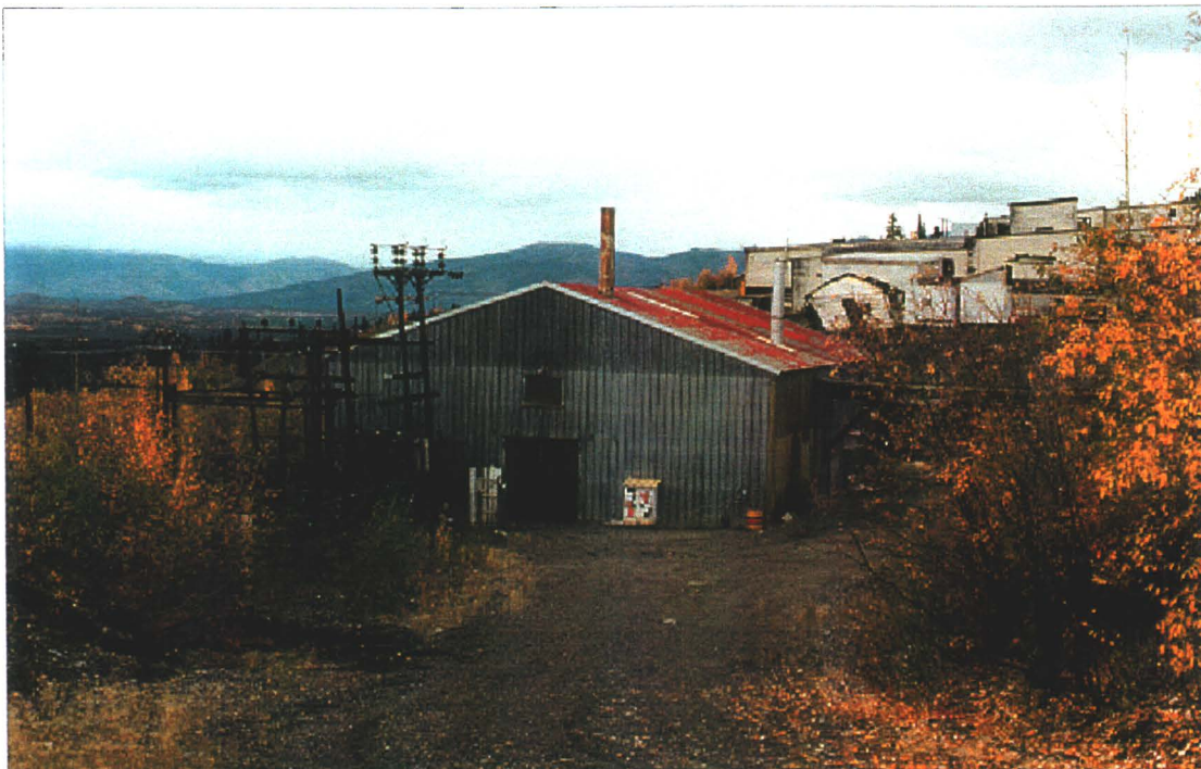
Photo 78-17 : Elsa. The boiler plant with an electrical substation beside it, the mill in the background. (Azimuth 020° )
