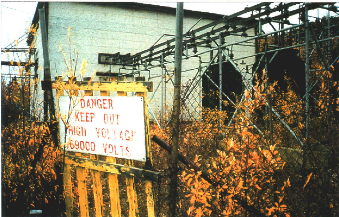
Photo 78-50 : Elsa. Electrical Equipment Area #5, transformers beside the adit portal.
