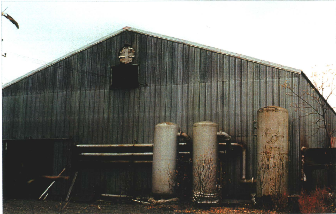
Photo 78-16 : Elsa. View of the vessels on the north end of the boiler plant (Building #21). (Azimuth 200° )
