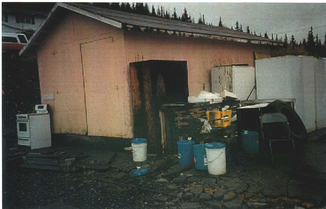
Photo 78-35 : Elsa. Storage shed below mine houses. Note pails full of waste oil. (Building # 52)
