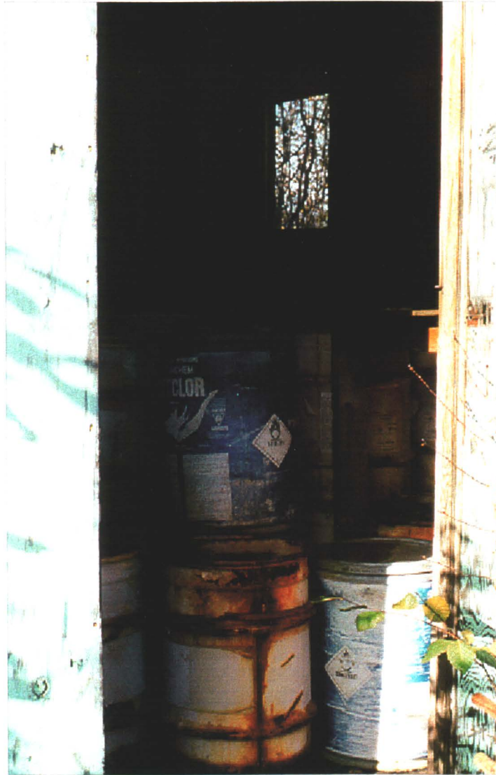
Photo 78-2 : Elsa. Building #1 is being used to store pails of calcium hypochlorite. (Azimuth 360°)
