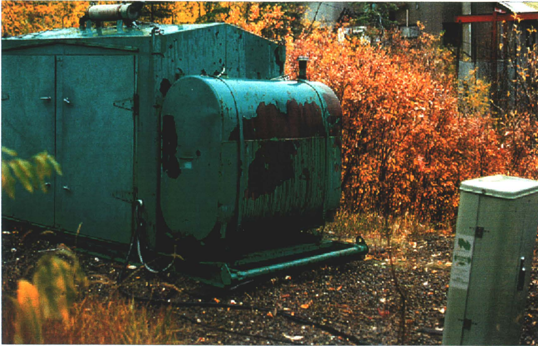
Photo 78-49 : Elsa. Electrical Equipment Area #4b - a mobile generator beside the Norwest Tel Building. (Azimuth 200°)
