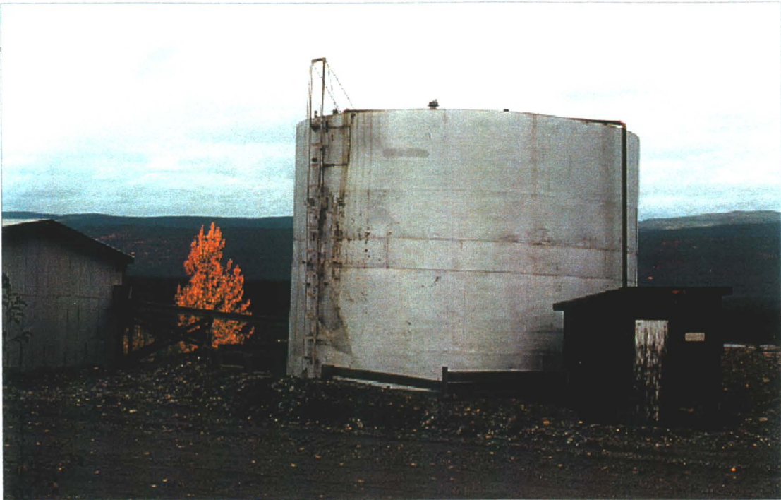
Photo 78-40 : Elsa. Fuel Storage Area #3 - an oil storage tank located beside the rescue building. There are numerous oil stains around the tank. (Azimuth 290°)
