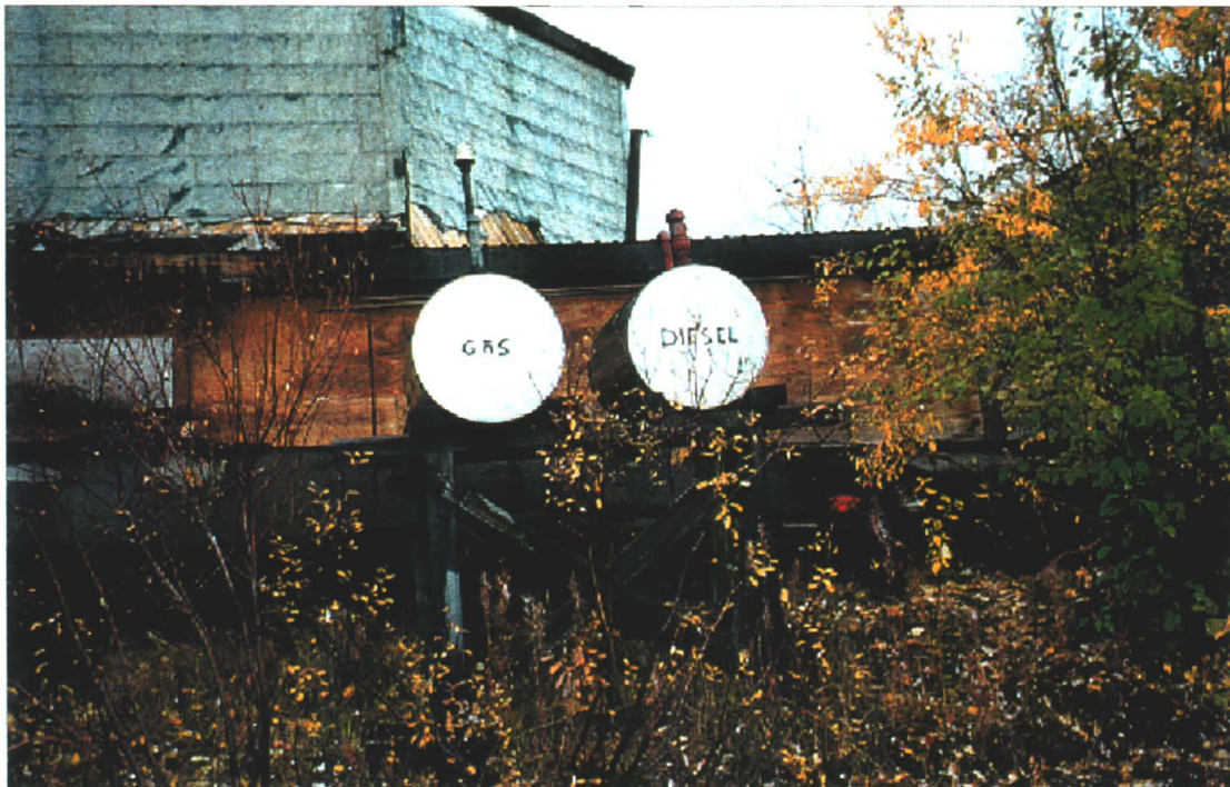
Photo 78-44 : Elsa. Fuel Storage Area #7, these two ASTs are located on the north side of the Mill (Building #20).
