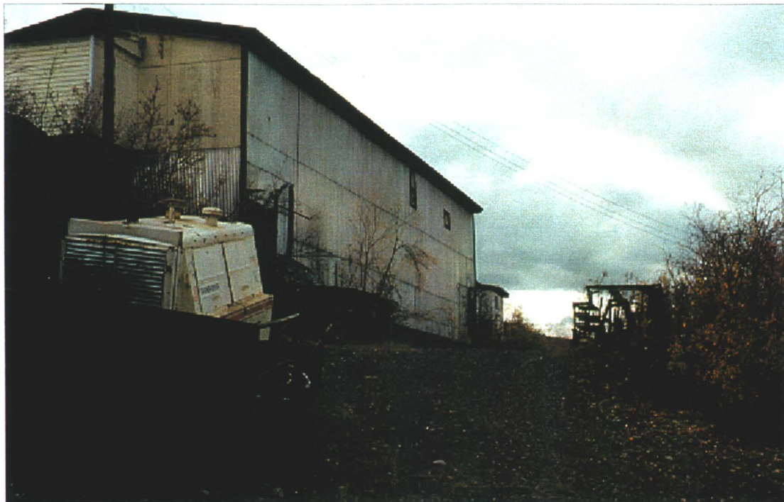
Photo 78-48 : Elsa. Electrical Equipment Area #4a - a mobile generator parked behind the Elsa Market. (Azimuth 230°)
