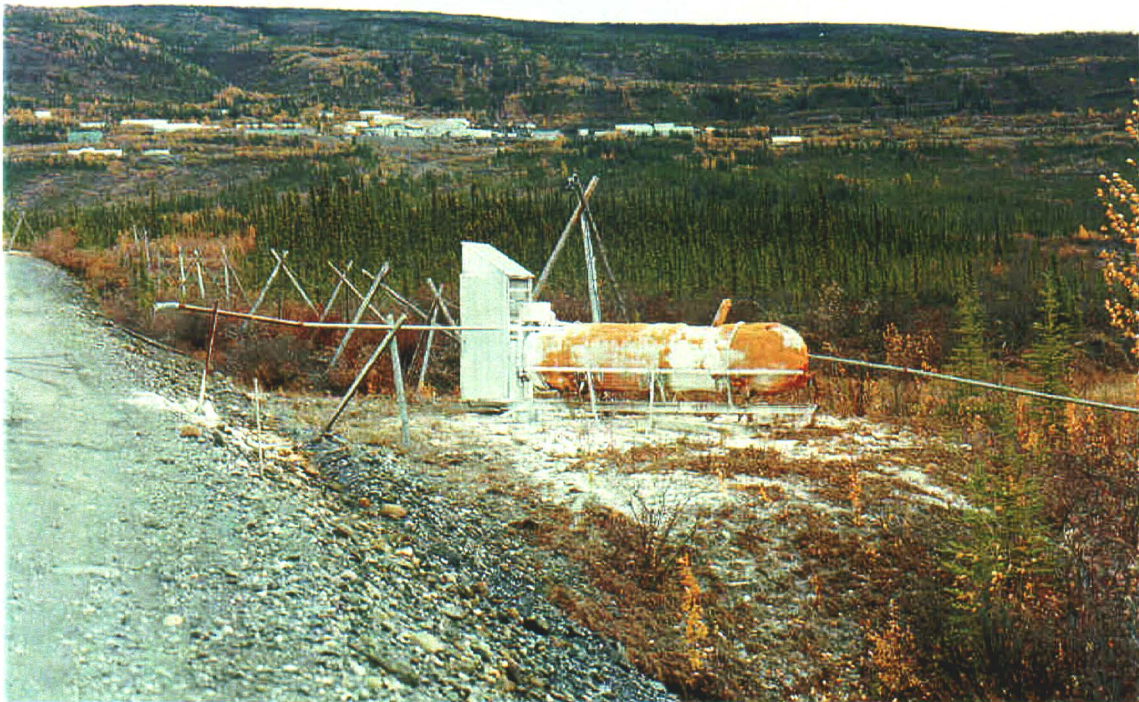
Photo 79-16. Lime treatment plant on Dam No. 2.
