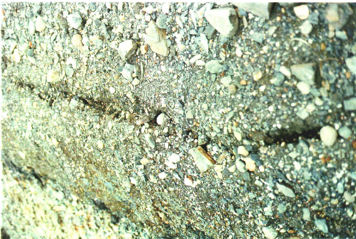
Photo 79-6. Tension cracks in tailings Dam No. 2.
