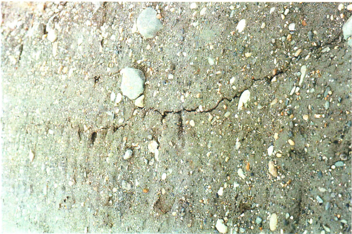
Photo 79-12. Tension cracks in Dam No. 3.
