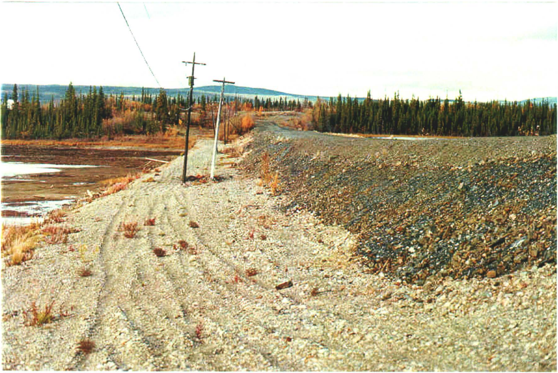
Photo 79-1. Toe berm (light-colored material) at the base of Dam No. 1, looking northwestward.
