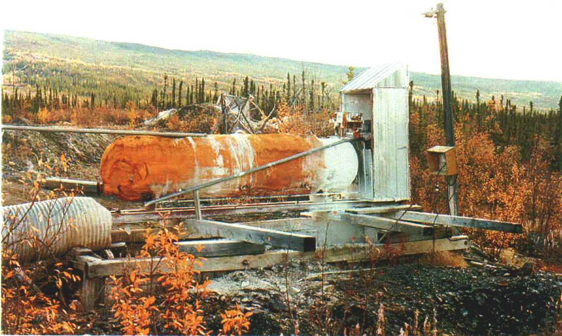
Photo 79-15. Lime treatment plant on Dam No. 1.
