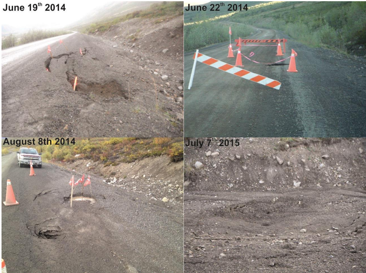
Figure 3.1.1 Degradation observed at site DH82 in 2014 and 2015.
