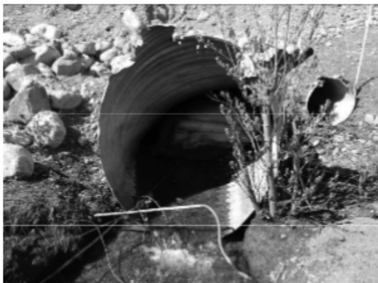
Figure 7. Culvert at km 32.5 (North Klondike River valley), filled with icing, May 2014. Photo by C.R. Burn.
