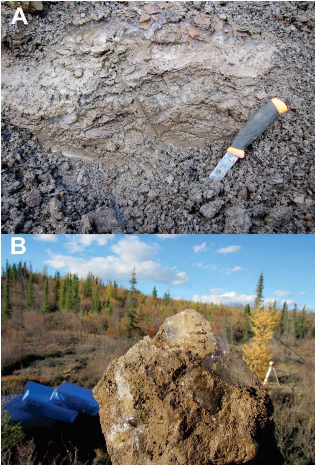
Figure 3.10.4 Permafrost observed during culvert installation at site DH381. A- ice-rich fine grained soil excavated below the embankment; B- close-up of an ice-rich permafrost sample collected during the excavation works
