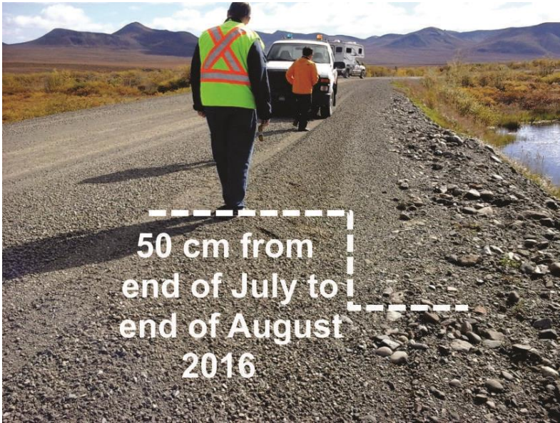
Figure 3.4.1 Subsidence observed at site DH103.
