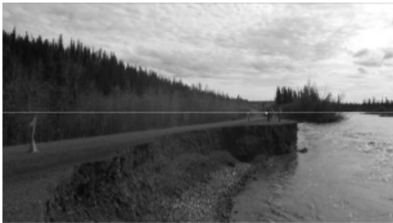
Figure 10. Wash out of the road by Ogilvie River at km 245, June 2013. Photo by S.N. Orban
