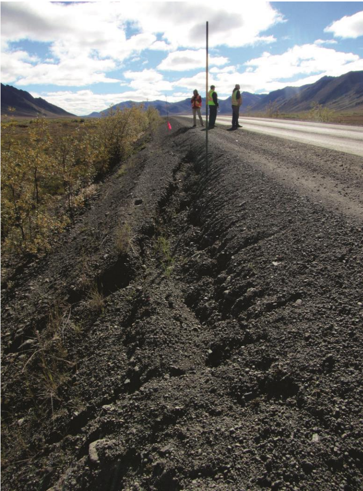
Figure 3.2.1 20m failure located on the RHS of the road at site DH95.
