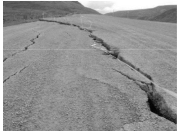
Figure 11. Thaw subsidence of the embankment at NT km 27, August 2011. Photo by C.R. Burn.
