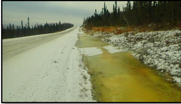
Figure 6. Groundwater-induced icing near km 29 on October 28, 2022.
