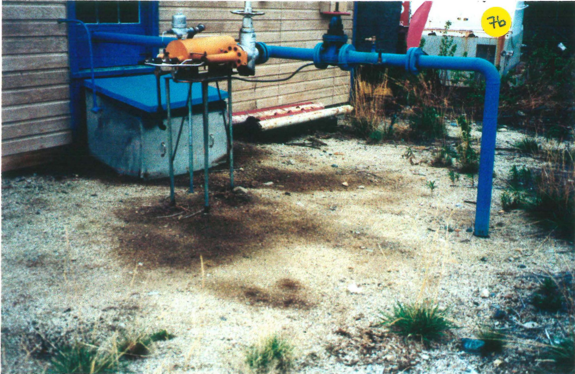
3.7b: Soil Staining near Meter Building
