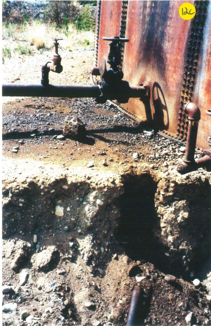
3.12c: Soil Staining at Tank 124
