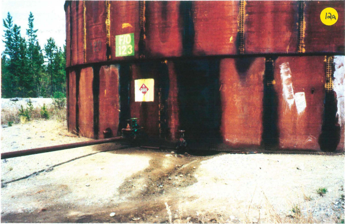
3.12a: Soil Staining at Tank 123
