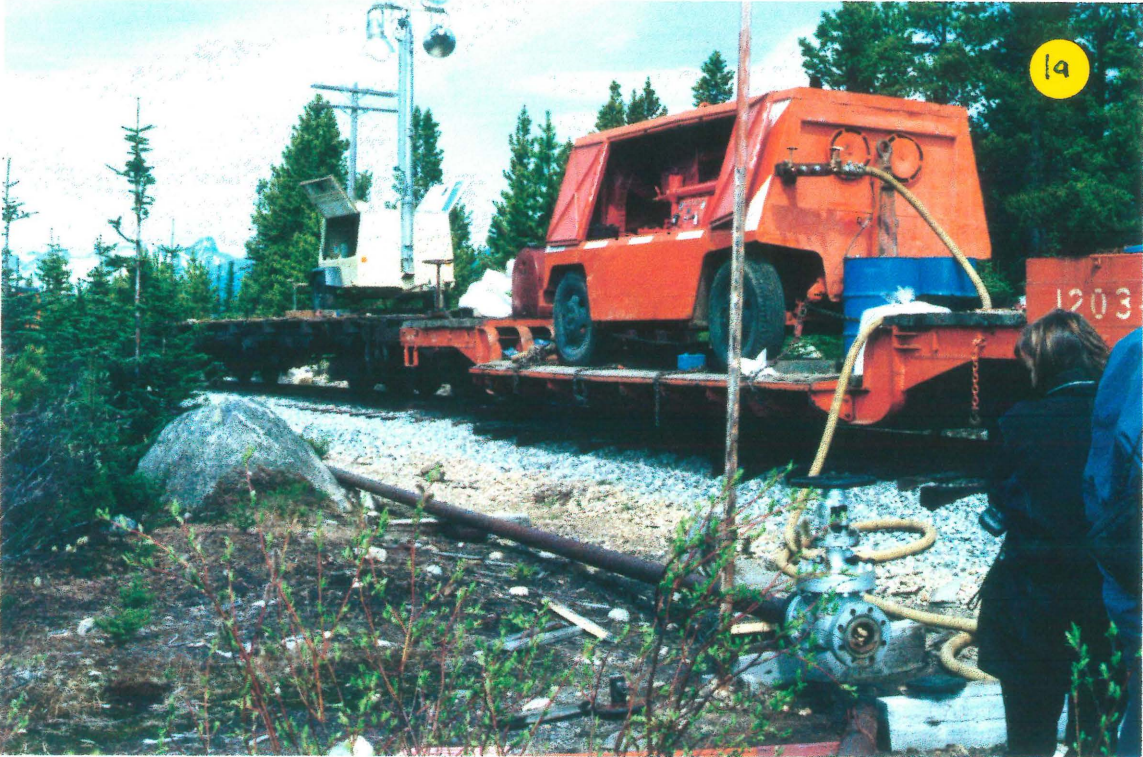
3.1a: Compressor for Pigging Pipeline
