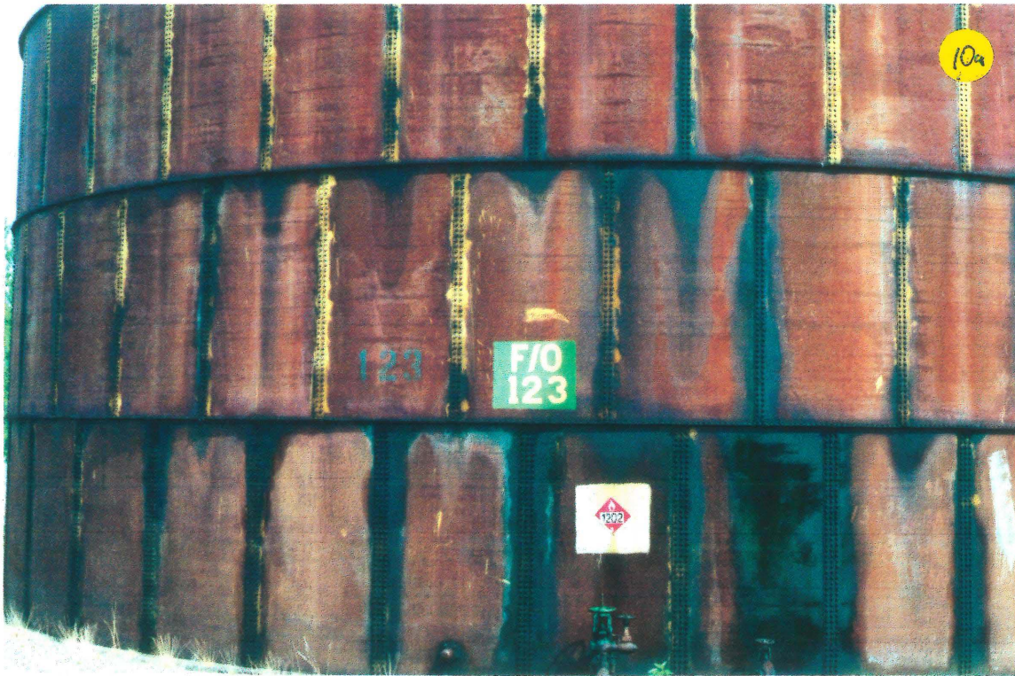
3.10a: Leakage from Tank Wall Seams
