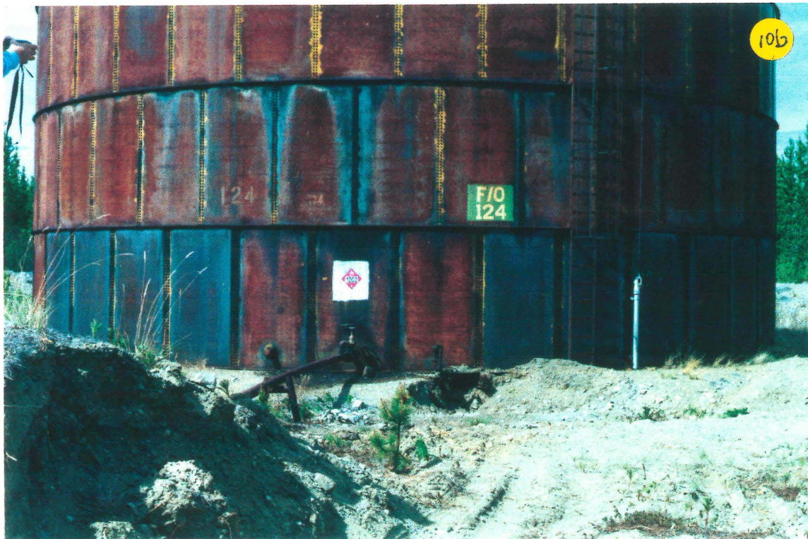
3.10b: Leakage from Tank Wall Seams
