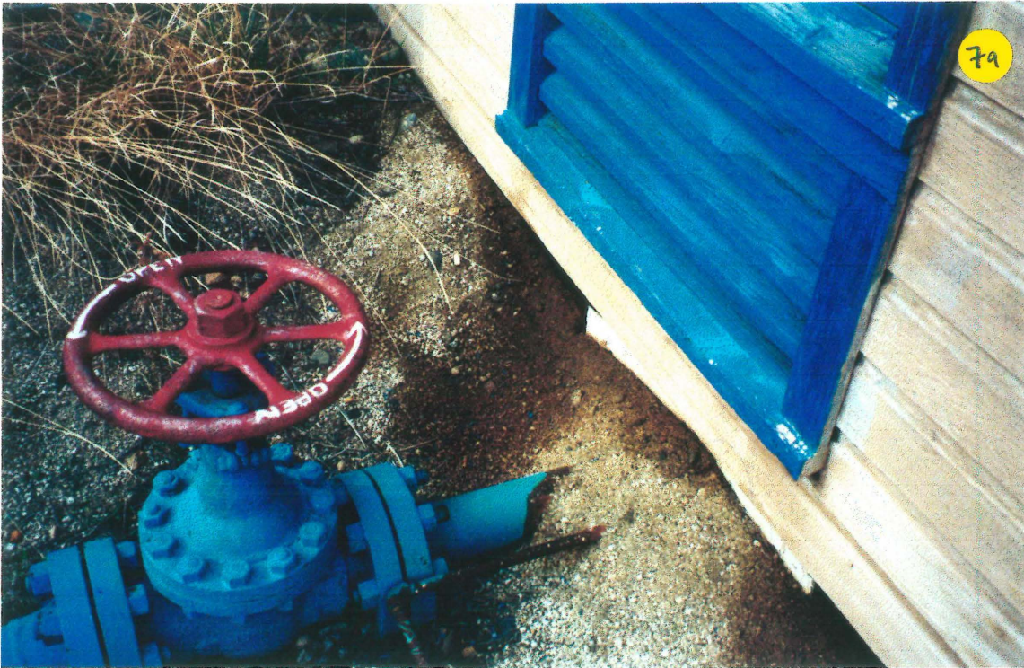
3.7a: Soil Staining near Meter Building
