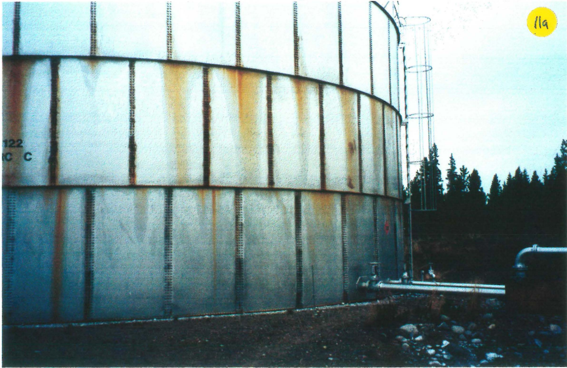
3.11a: Soil Staining at Tank 122
