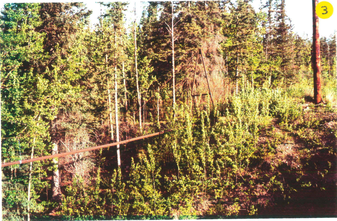
3.3: Pipeline and Support over Creek, Alaska Highway kmp 1470
