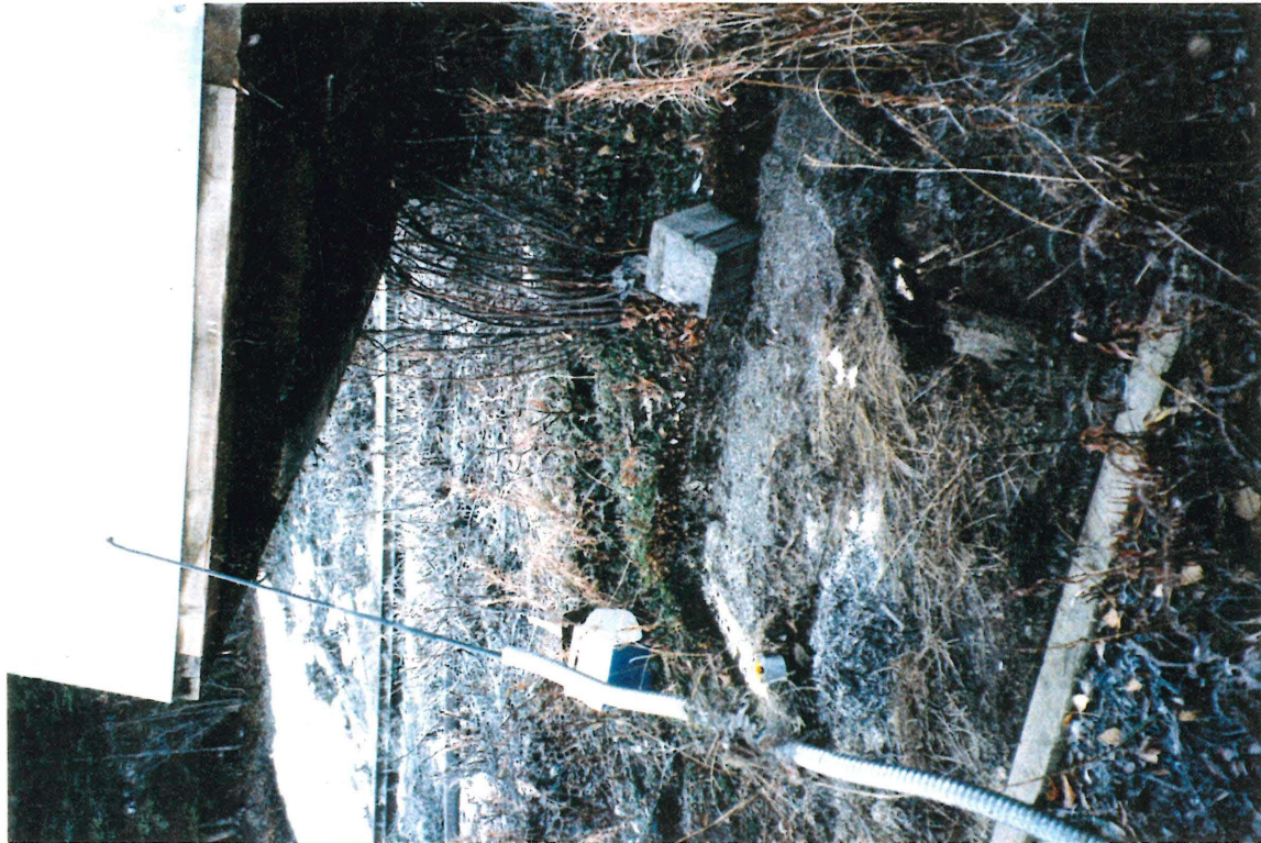
Photo C: Exposed soil under building
