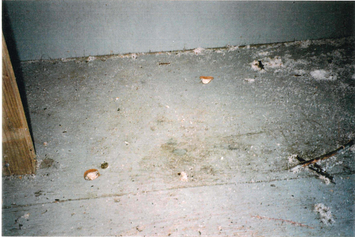
Photo E: Holes in floor of building
