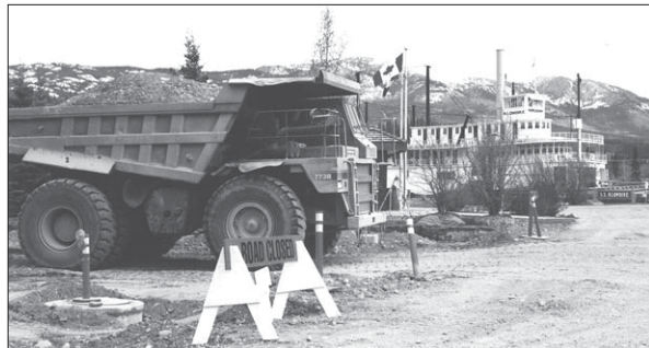
Construction of a new parking lot in partnership with the City of Whitehorse, 1997
