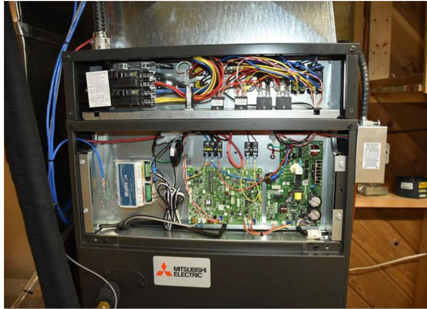
Figure 7: Inside of the indoor cold-climate heat pump unit and the backup auxiliary heat with the power monitoring.
