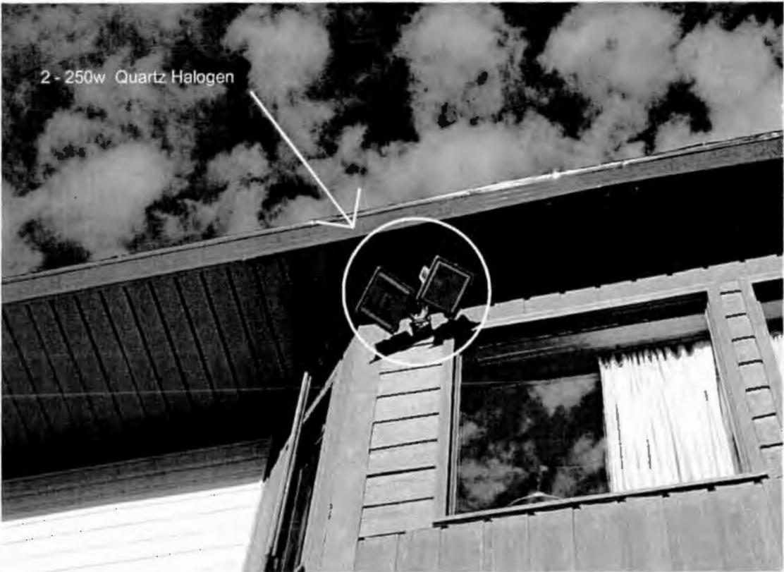
Photograph Five Outside 250W quartz halogen to be replaced with 70W high pressure sodium.
