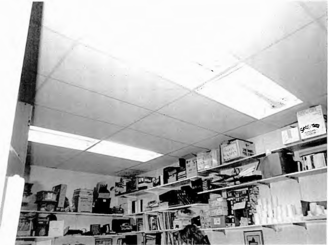
Photograph Six Office 4 lamp T12 fixture to be replaced with 2 lamp T8 fixture.
