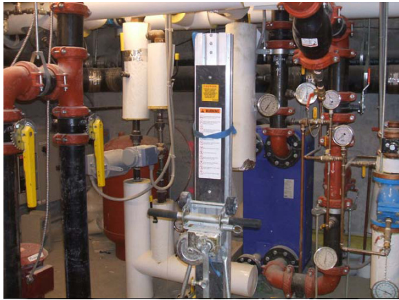
Figure 10: Energy Transfer Station Installation
