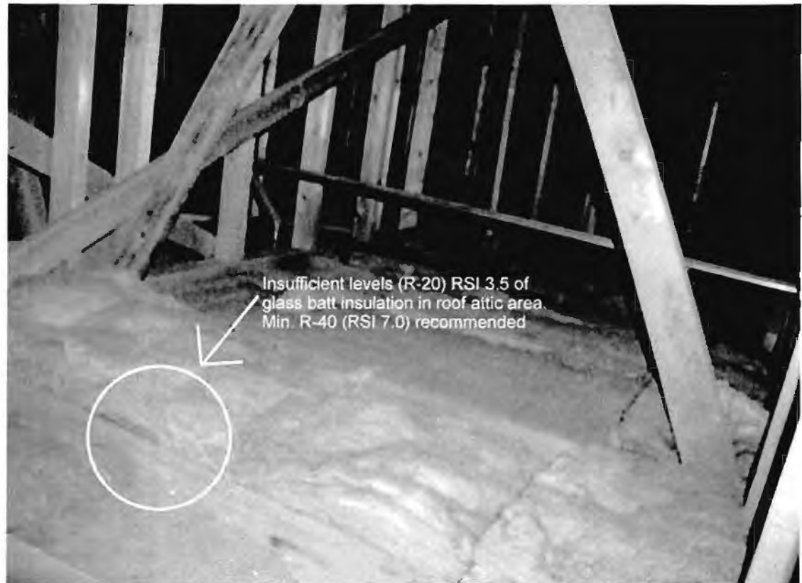
Photograph Nine Roof attic - Insufficient levels of glass fibre batt insulation.
