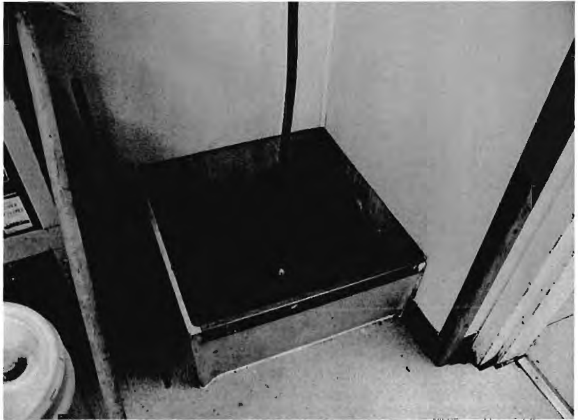
Photograph Eleven Hot water losses due to leaking tap at janitor mop sink
