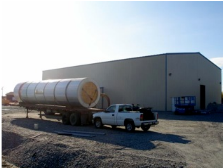
New Superior Pellet mill in Fairbanks, rotary dryer in front, about to be installed.
