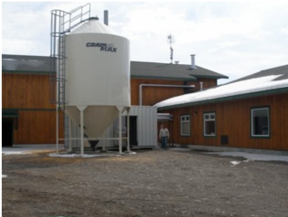
Recently converted Nazko Elementary School in BC, replacing propane with wood pellets using Viessmann KOB Boiler
