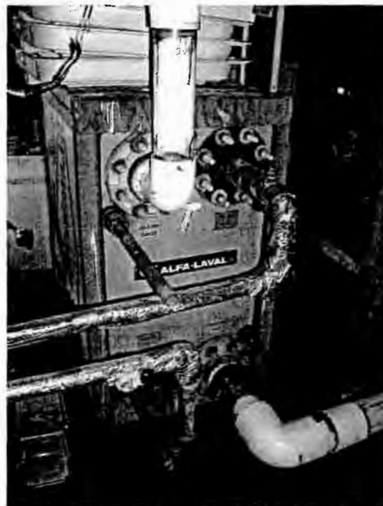
Figure 6 Existing Alpha-Laval Heat Exchanger
