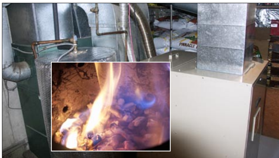
This combination of a wood pellet furnace with a backup oil furnace is a good heating setup for the owners who like the steady, even heat from wood. The pellet furnace burns very cleanly and generally requires little maintenance apart from daily loading of pellets. The pellets are made of sawdust-sized wood particles. The resin in the wood liquifies under pressure, binding and forming the pellet. Pelletizers can use a variety of sawmill wastes, so long as bark is a very small proportion (less than 5%) of the feed material. Peter Long
