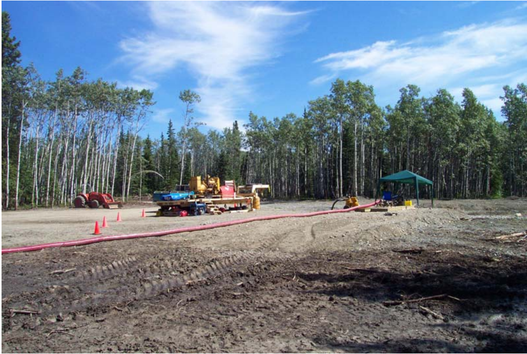
Photograph 2: Set-up for pumping test. Note: Generator on trailer deck (left), trash pump beside wellhead, canopy over well head (right) and discharge line running northwest from wellhead.
