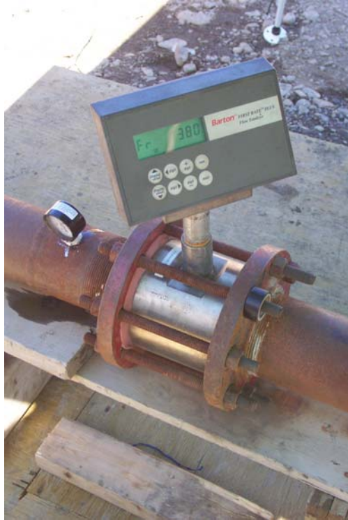
Photograph 6: Barton flow totalizer flow meter measuring instant and total flow during second step of pump test (380 Usgpm)
