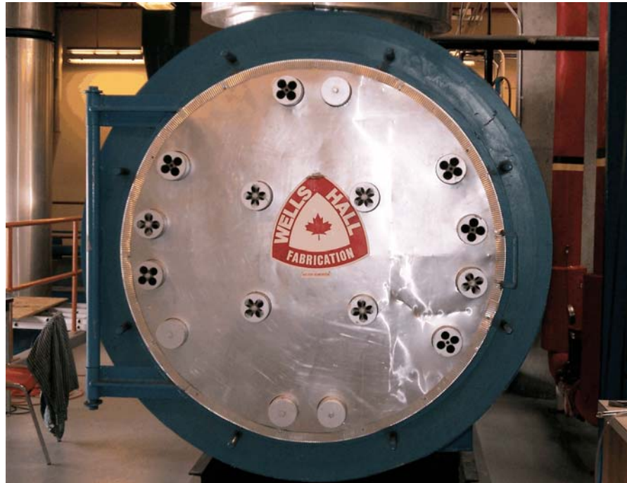
Figure 18. Back End (Exhaust) of B1 Boiler
