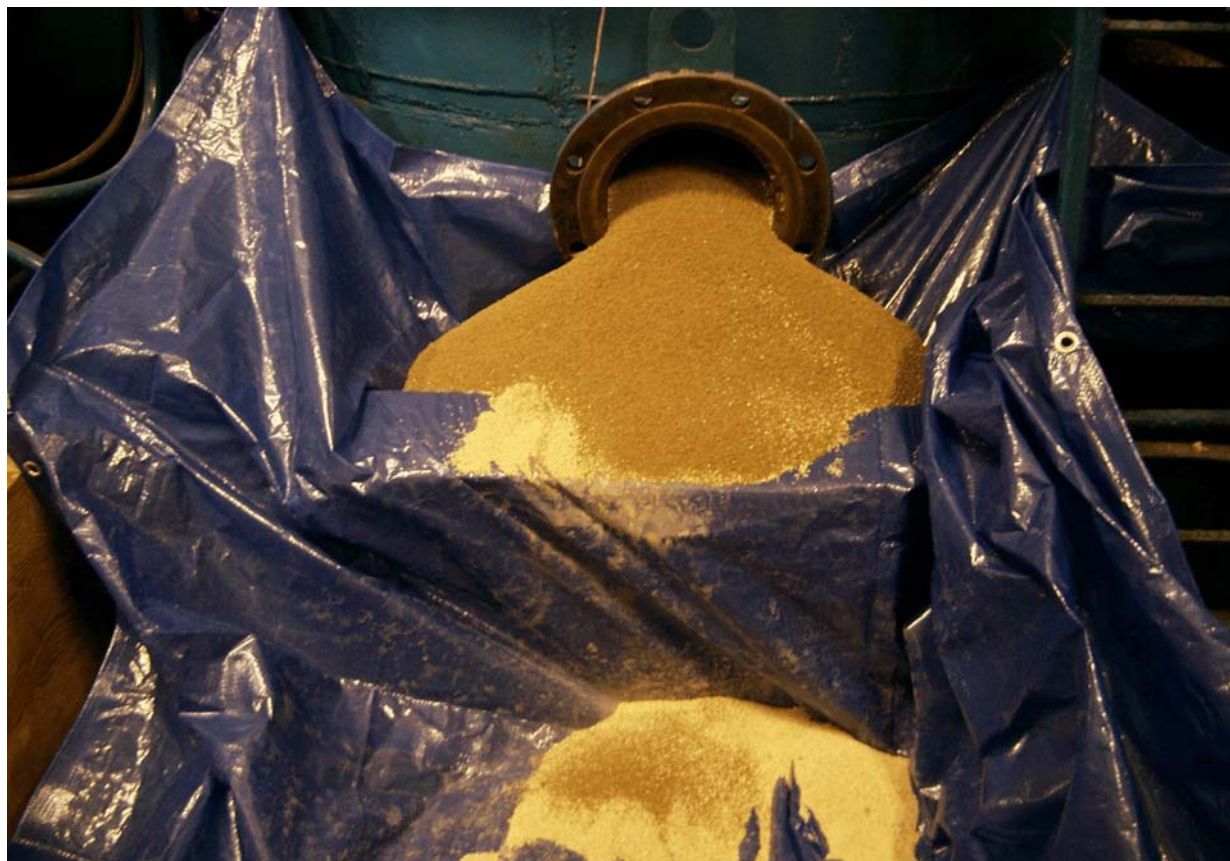
Figure 8. Sand removal port at bottom of gasifier
