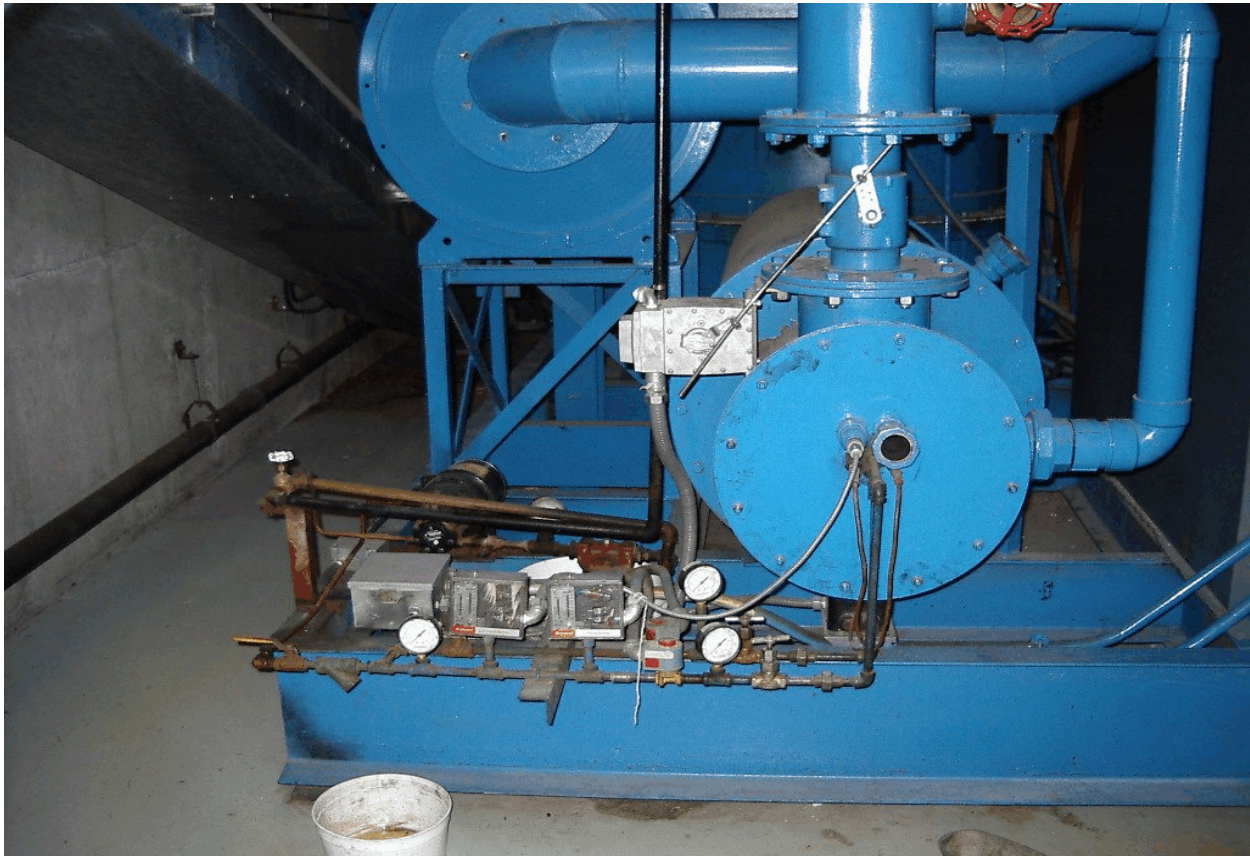
Figure 6. Oil-fired pre-heat system
