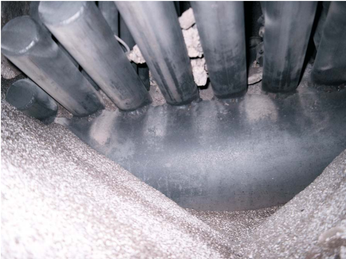
Figure 9. Air distribution system seen from ash removal port
