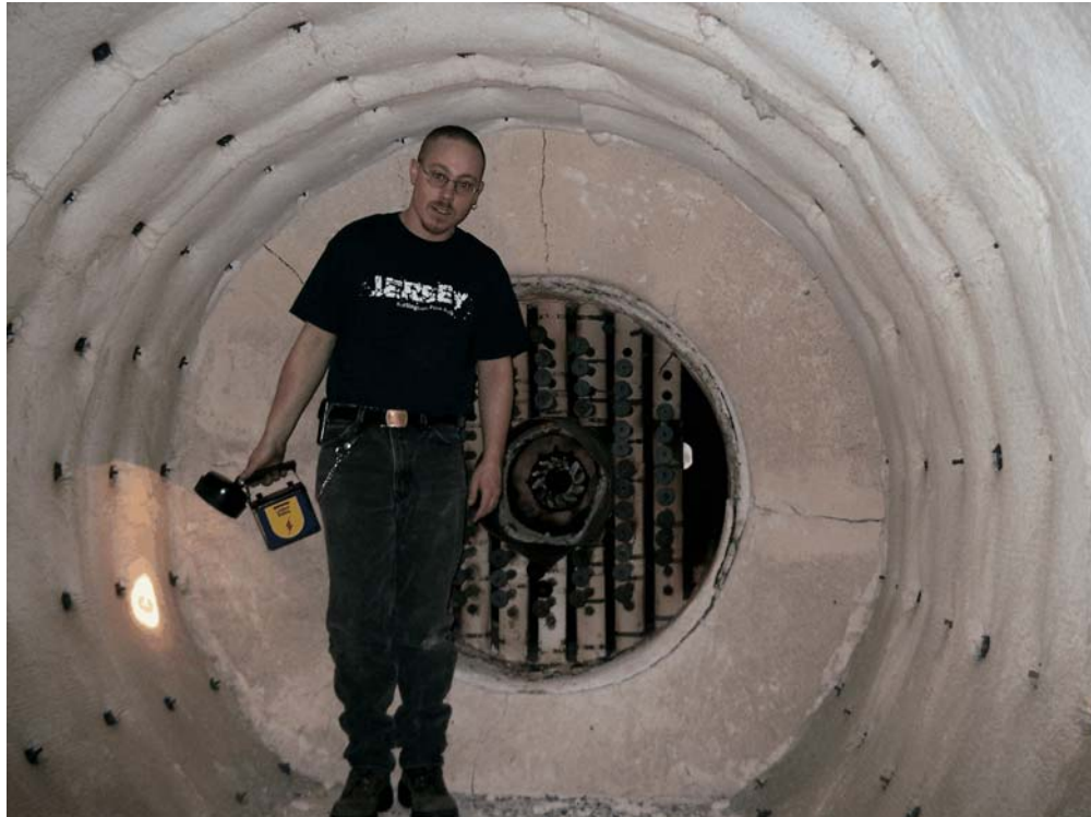
Figure 16. Interior of “Syngas” combustion chamber (B1 Boiler)
