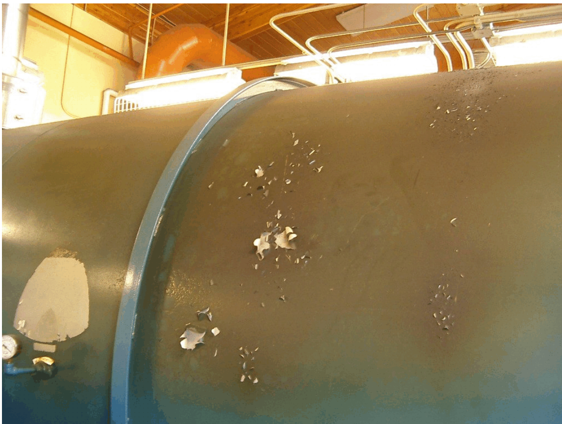
Figure 29. Damaged paint on B1 Boiler after gasifier test
