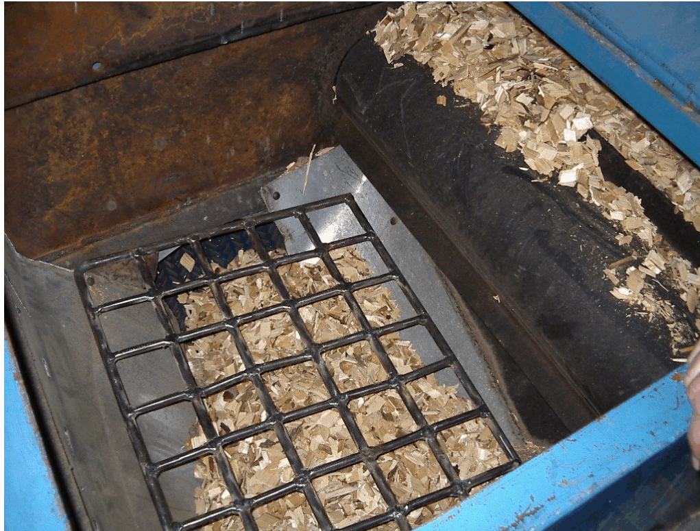
Figure 28. Steel grate installed to prevent jamming in feed system
