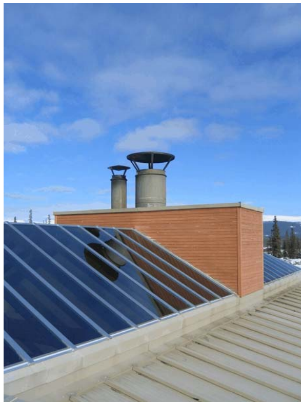
Figure 19. Stack of B1 Boiler/Gasifier RHS
