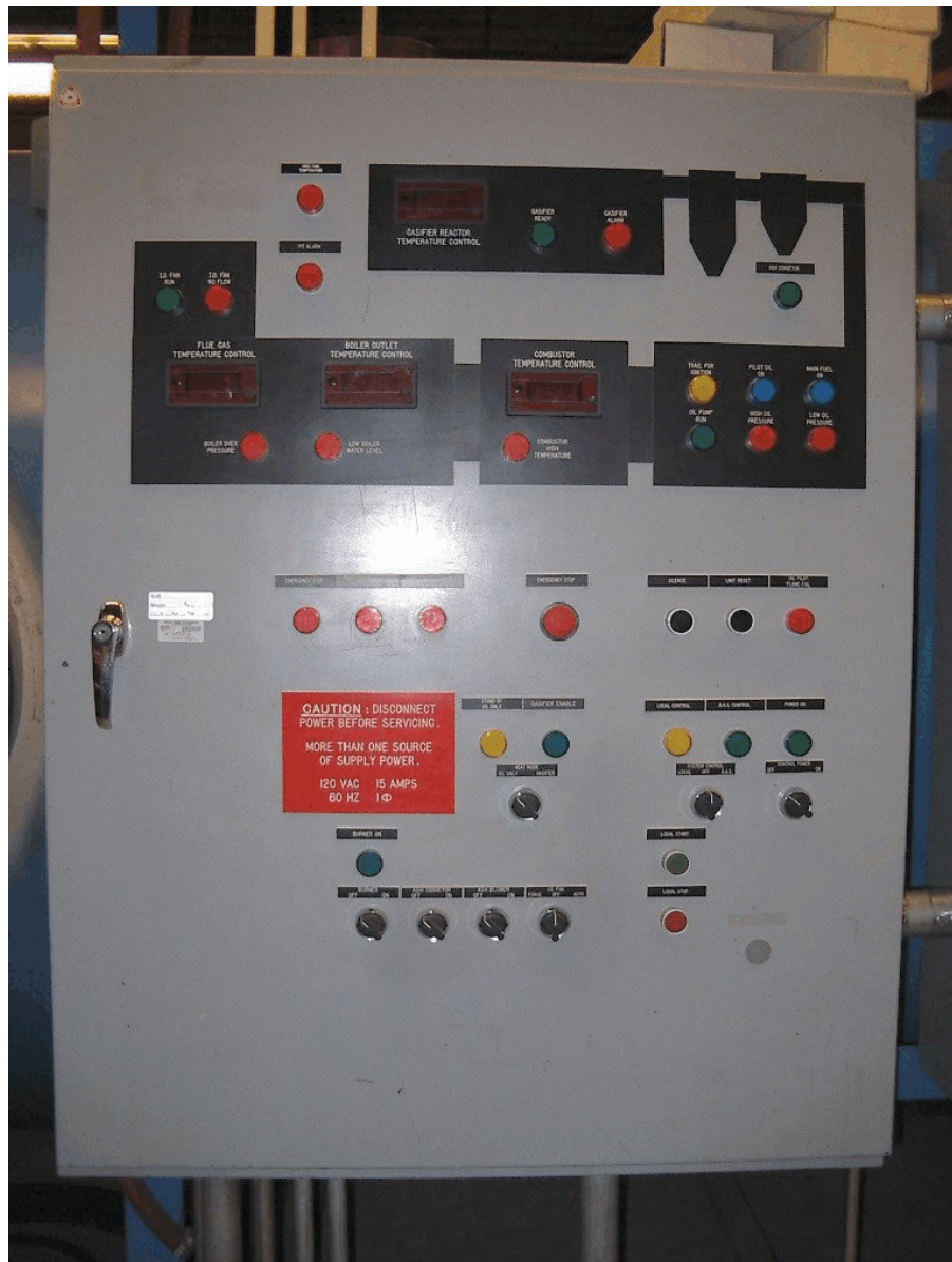
Figure 20. Existing Gasifier Control Panel
