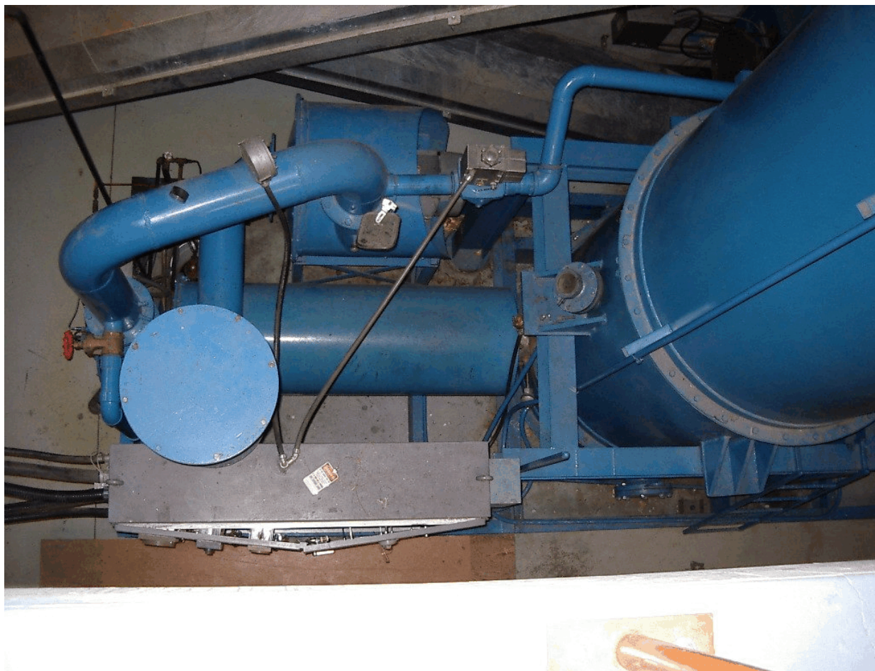
Figure 5. Air compressor and pre-heater seen from above
