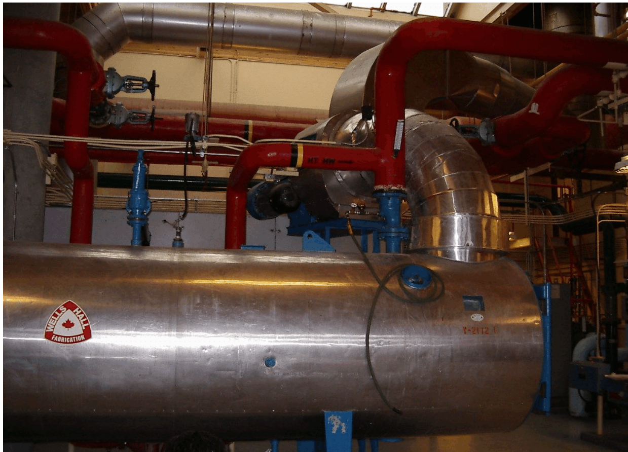
Figure 14. B1 fire tube boiler
