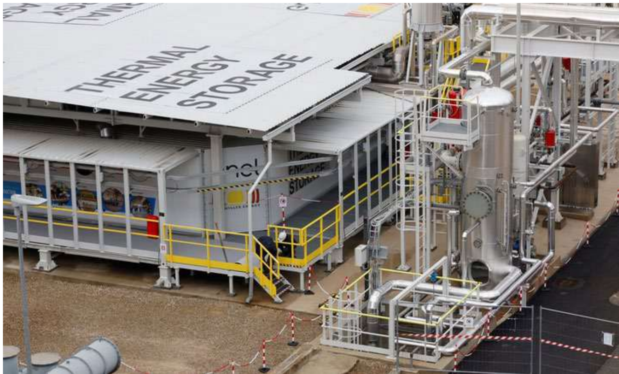
Figure 18: TES for power generation installed at Enel's Santa Barbara power station in Italy [29]
